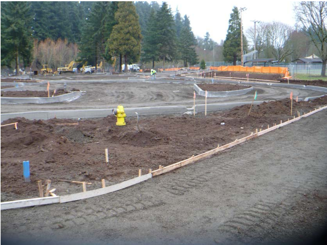
View looking north at perimeter sidewalk, parking lot extension, and new islands
