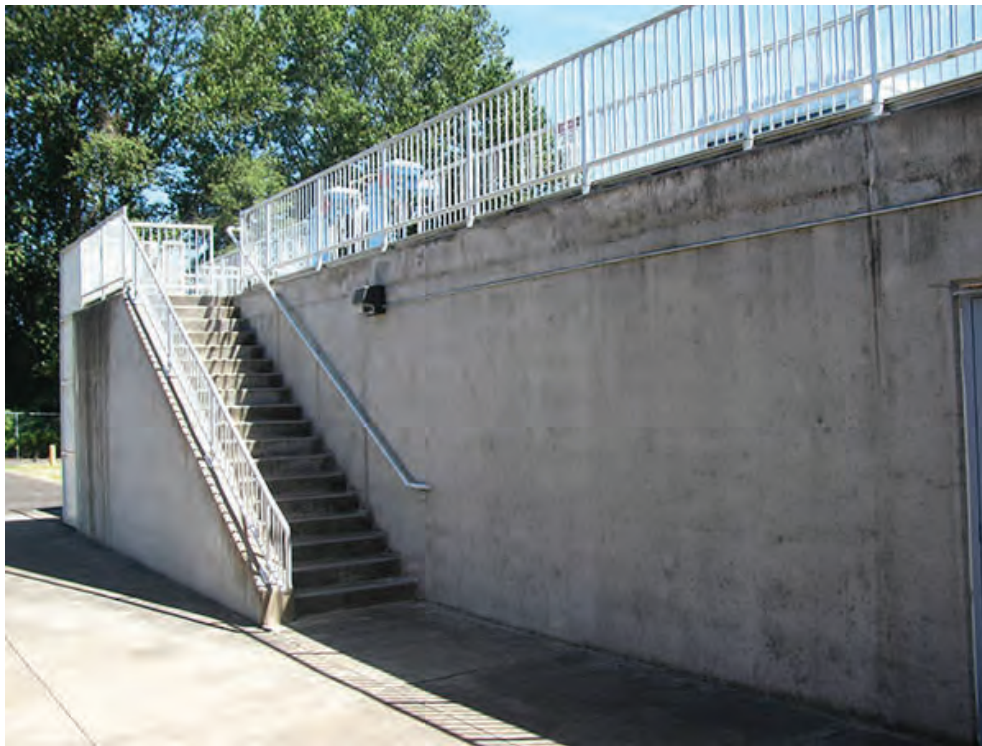
Photo 6 – LS3 – Guardrail at the north Filter staircase is less than 42 inches in height.
