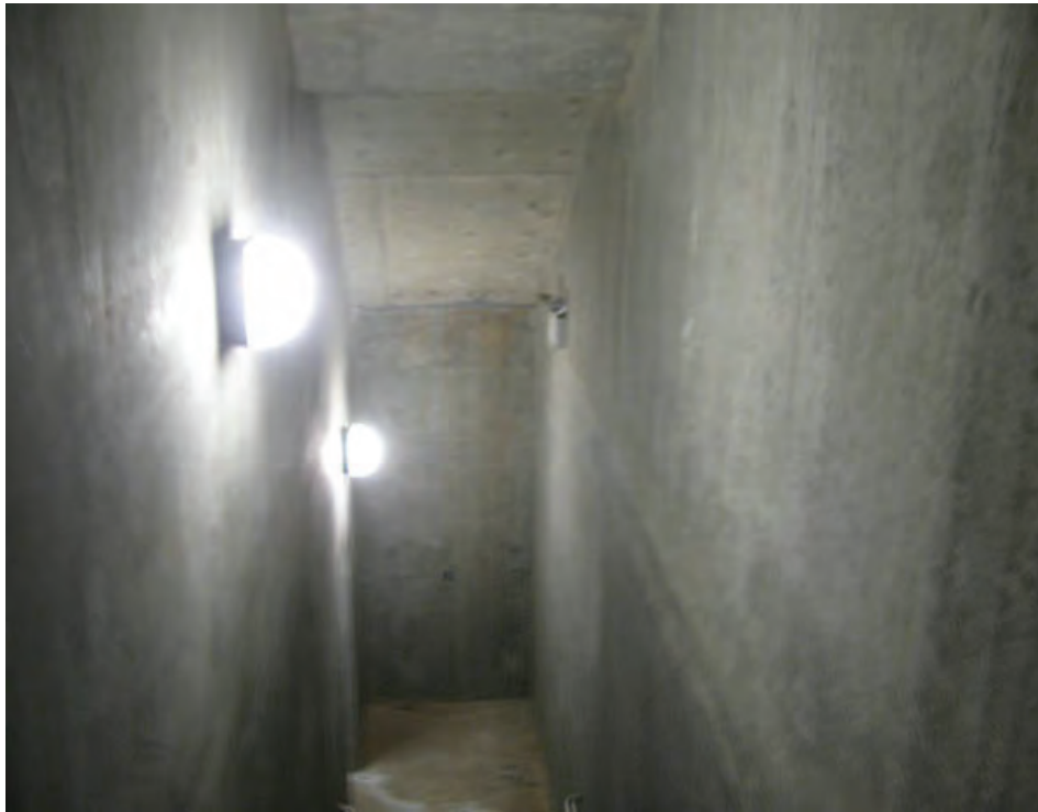
Photo 21 – LS11 – The south stairwell at the Ozonation Basin has no dedicated ventilation.
