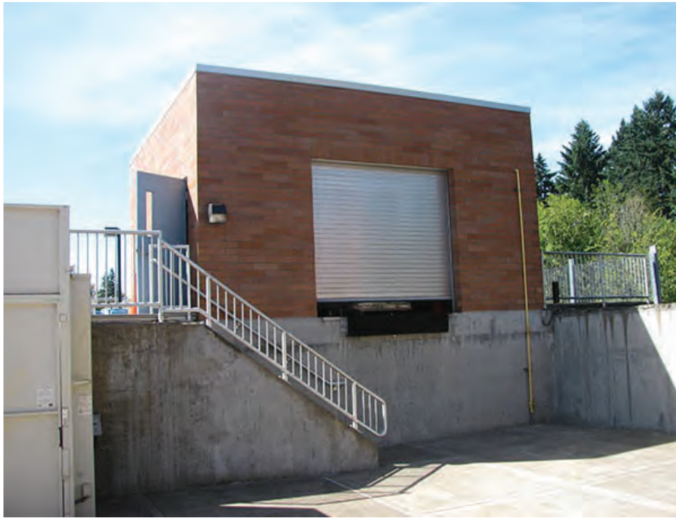
Photo 5 – LS3 – Guardrail at the north Actiflo™ staircase is less than 42 inches in height.
