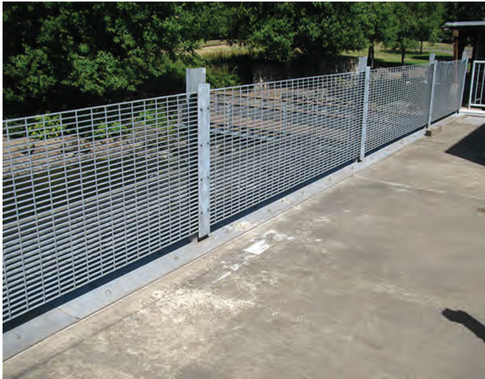
Photo 15 – LS8 – West guardrail on top of the Actiflo™ Basin lacks a kick plate and it is located over a public walkway.
