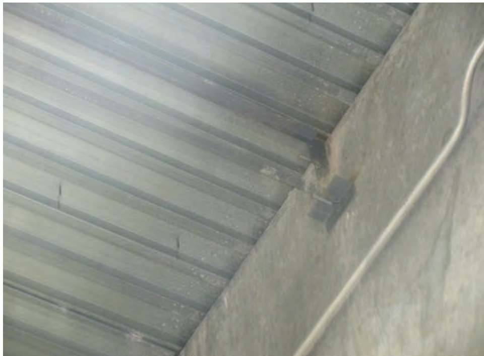
Photo 30 – S6 – Interior walls lack diaphragm shear capacity transfer from the roof diaphragm to the shear walls.
