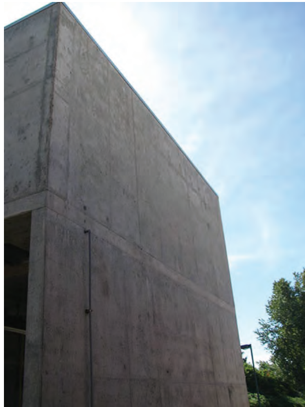
Photo 26 – LS14 – The Solids Dewatering Building does not have any overflow scuppers visible.
