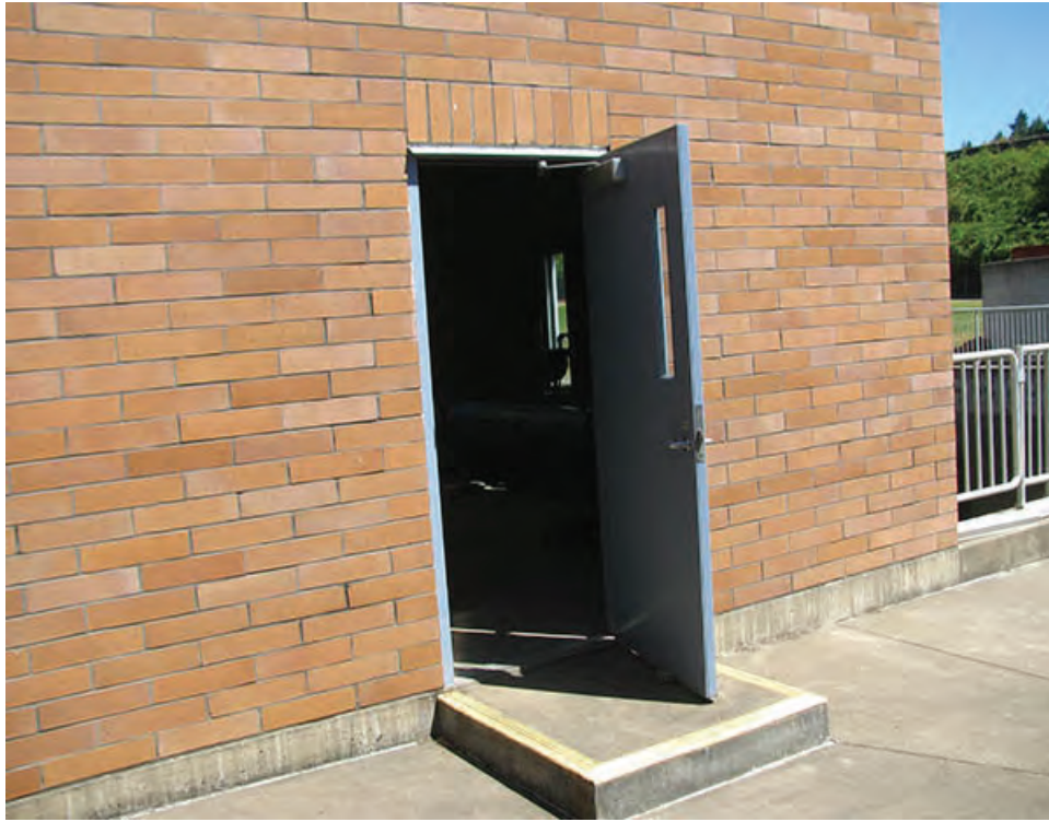
Photo 13 – LS7 – Door at the Waste Washwater Pump Station was found propped open.
