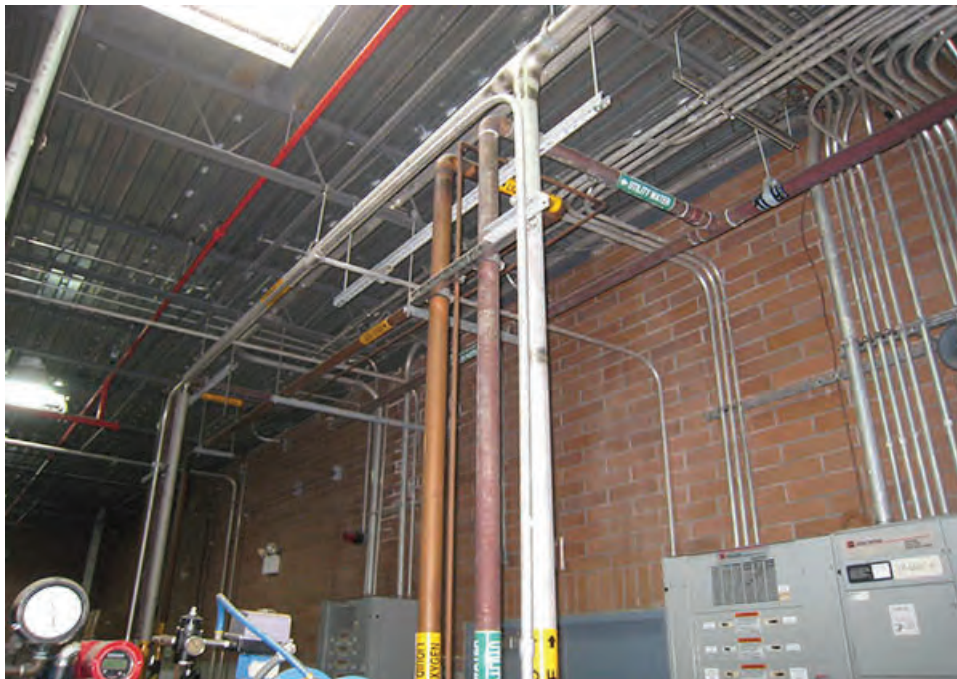
Photo 38 – S14 – The ozone and LOX piping at the Ozone Generation Room lacks seismic bracing.
