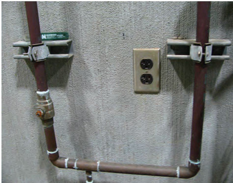
Photo 19 – LS10 – Standard electrical receptacle inside the Ozone Gallery.
