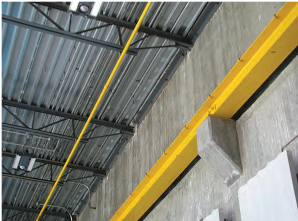
Photo 28 – S3 – The roof joist wall anchorage to the walls at the High Service Pump Station lack capacity to meet seismic performance goals.
