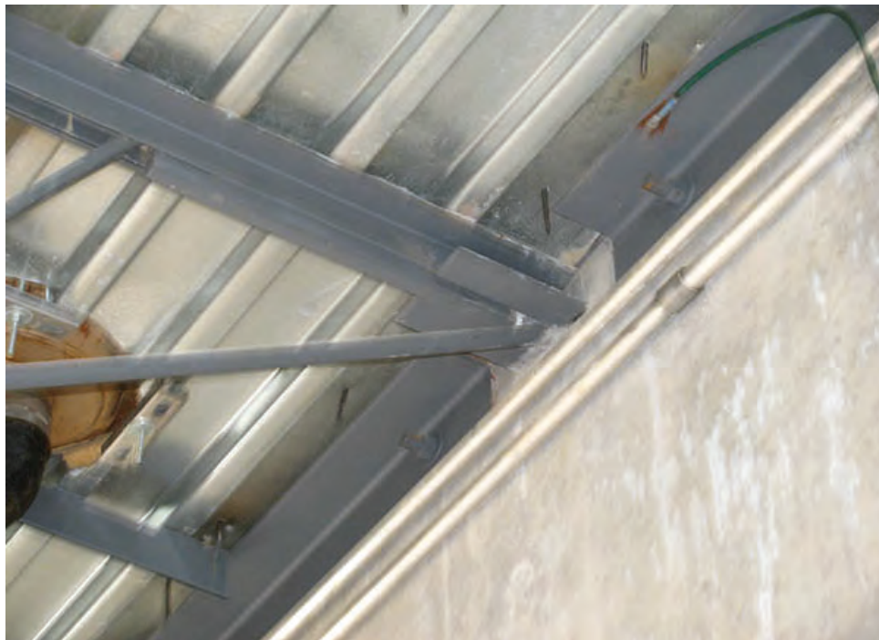
Photo 32 – S8 - The roof joist wall anchorage to the walls at the Solids Dewatering Building lack capacity to meet seismic performance goals.
