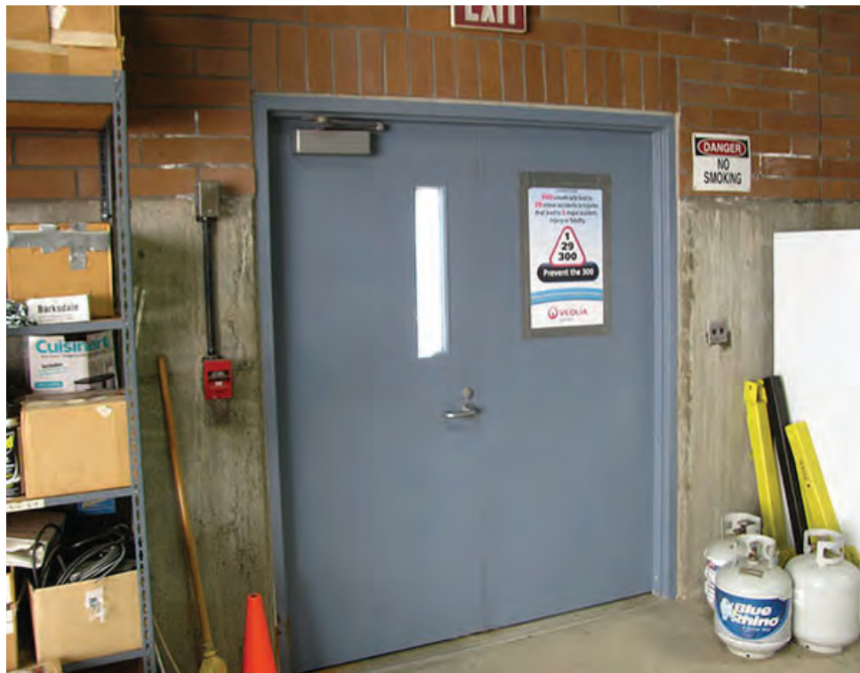
Photo 9 – LS5 – Group occupancy H at the Ozone Generation Room requires panic hardware on the exit doors (one of the south doors shown).
