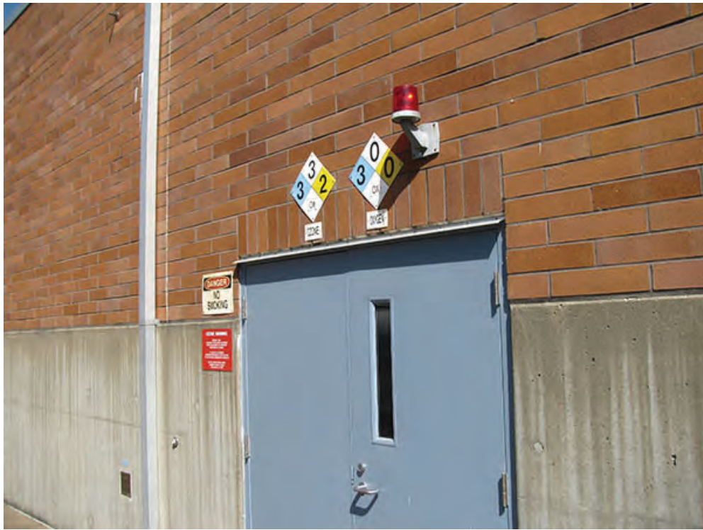
Photo 3 – LS2 – Color coded safety warning signs are faded at the south wall of the Ozone Generation Room.
