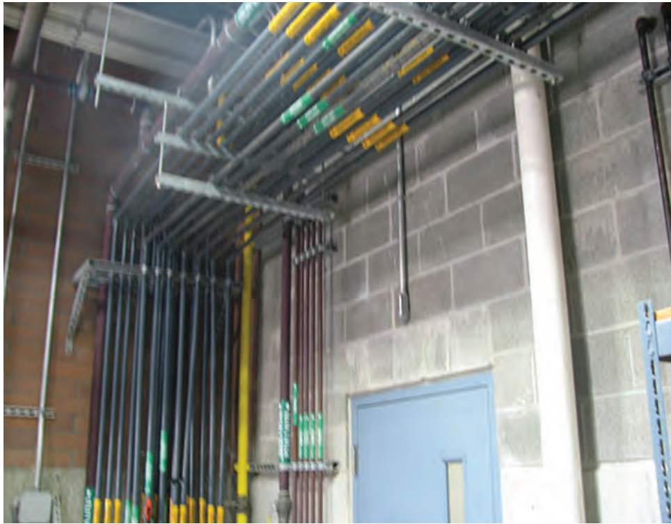
Photo 11 – LS6 – Chemical piping passing directly over the west door at the Ozone Generation Room.
