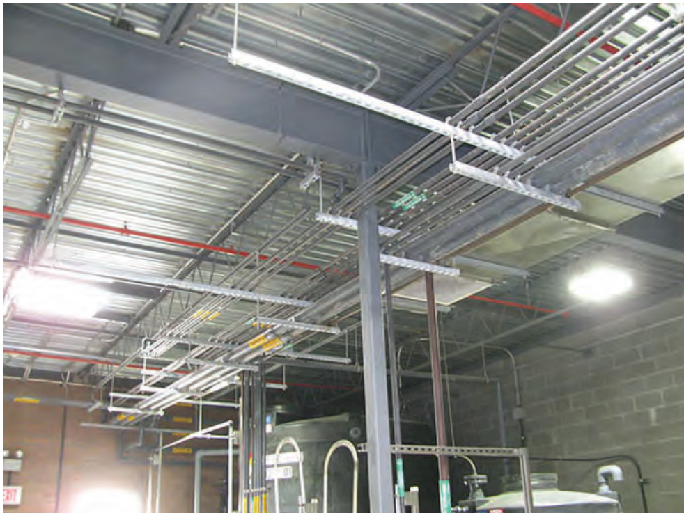
Photo 12 – LS6 – Chemical piping passing directly over the egress route to the east door at the Chemical Storage Room.
