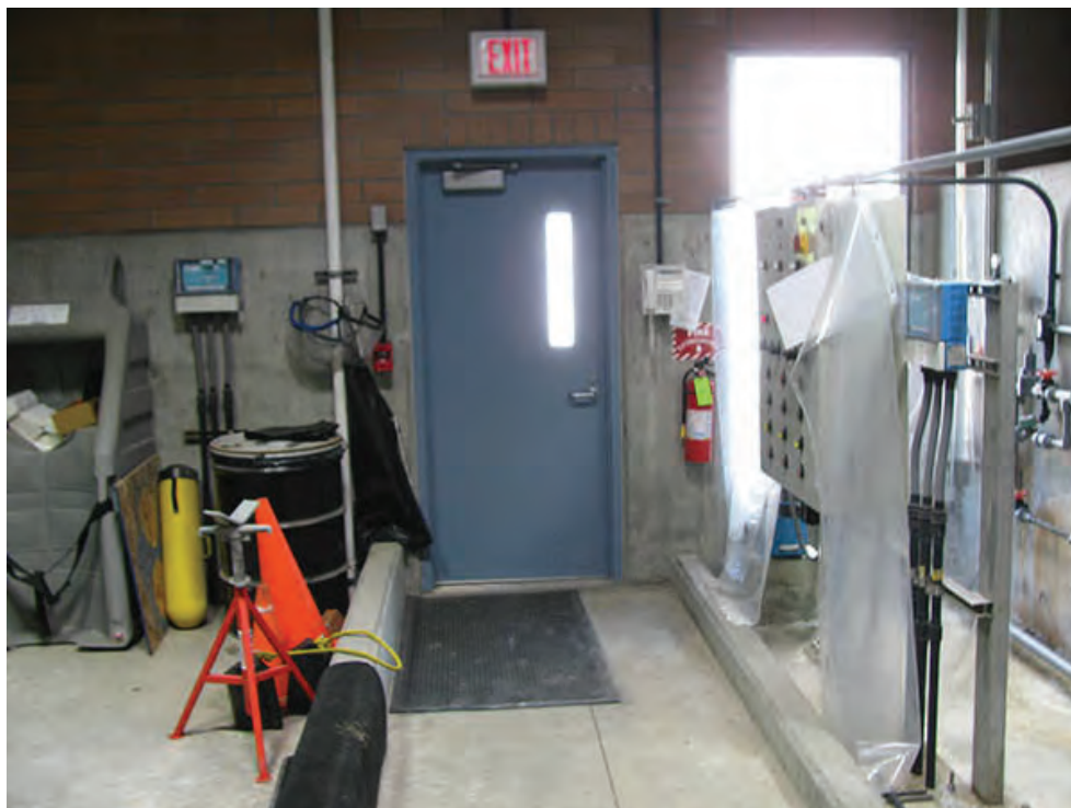
Photo 10 – LS5 – Group occupancy H at the Chemical Storage Room requires panic hardware on the exit doors (the east door shown).
