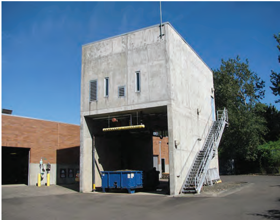
Photo 25 – LS14 – The Solids Dewatering Building does not have any overflow scuppers visible.
