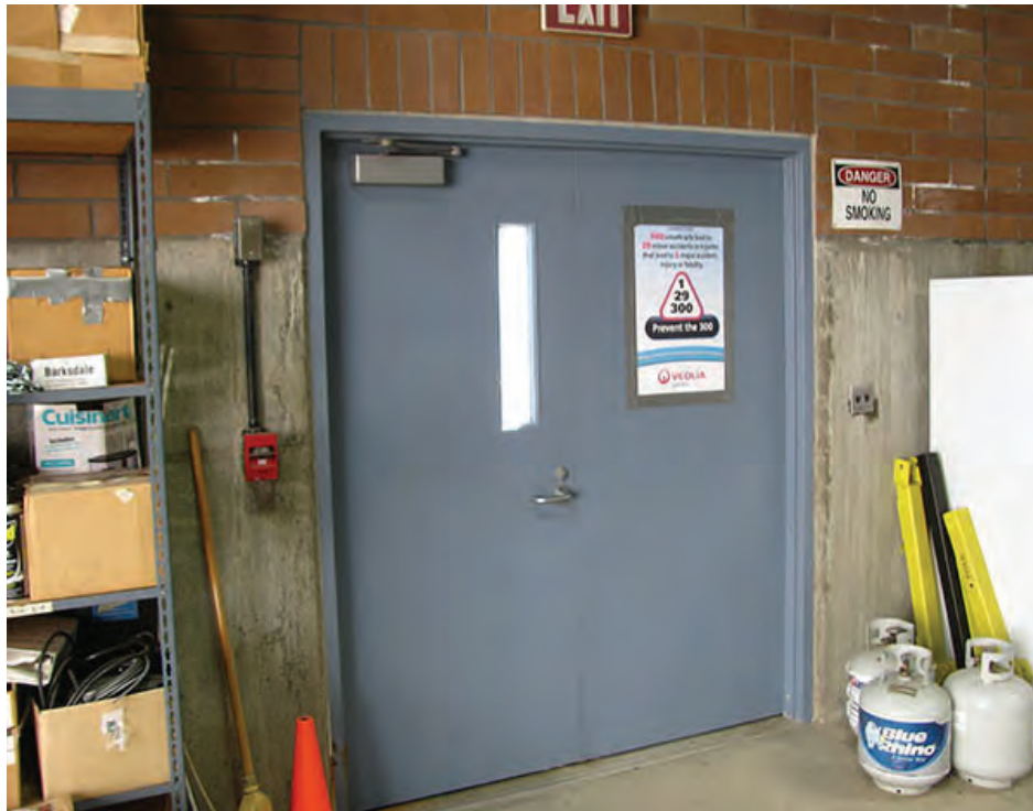
Photo 27 – LS15 – The southeast door that exits from the Ozone Generation Room does not have an emergency shut-off switch for the ozone generation equipment.
