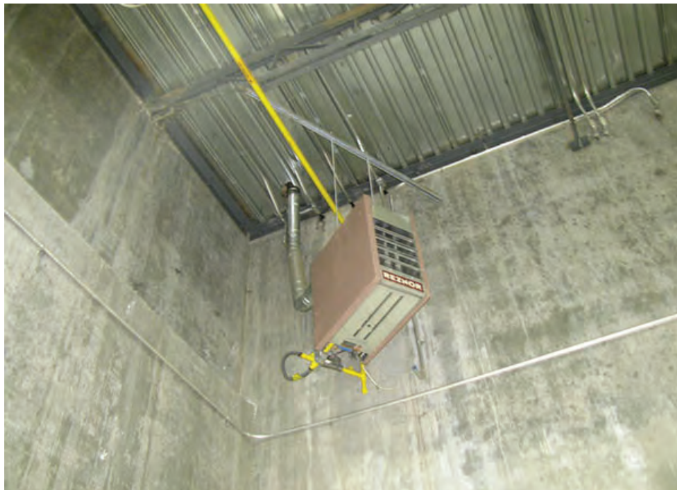
Photo 34 – S10 – The space heater at the Switchgear Room at the High Service PS is suspended without any seismic bracing.
