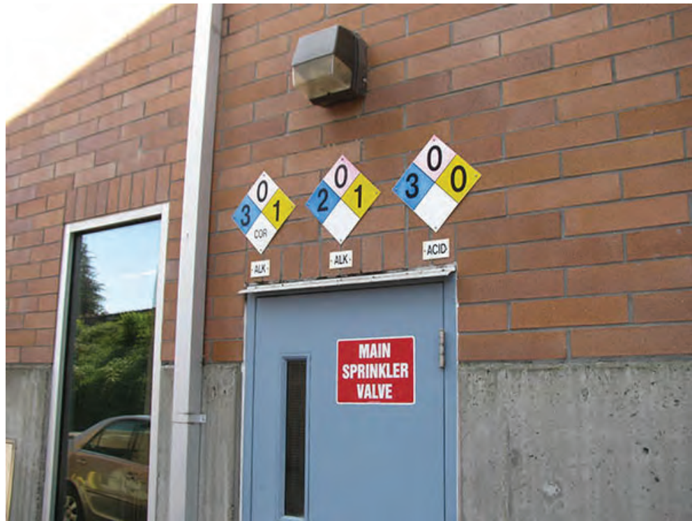
Photo 4 – LS2 – Color coded safety warning signs are faded at the east wall of the Chemical Storage Room.
