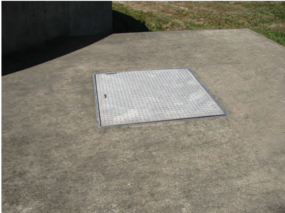
Photo 2 – LS1 – Access hatch at the Sludge Thickening PS as seen from the top side.
