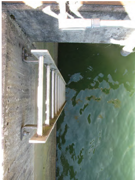
Photo 24 – LS13 – The access ladder to the Waste Washwater EQ Basin does not have any tie-offs for a fall restraint system.
