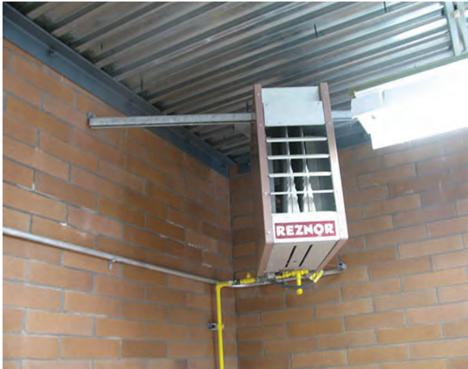
Photo 33 – S10 – The space heater at the Washwater Pump Station is suspended and unbraced for seismic loads.
