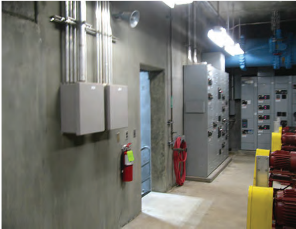
Photo 7 – LS4 – The Actiflo™ gallery has electrical service rated at 1200 amps or higher requiring panic hardware on doors.
