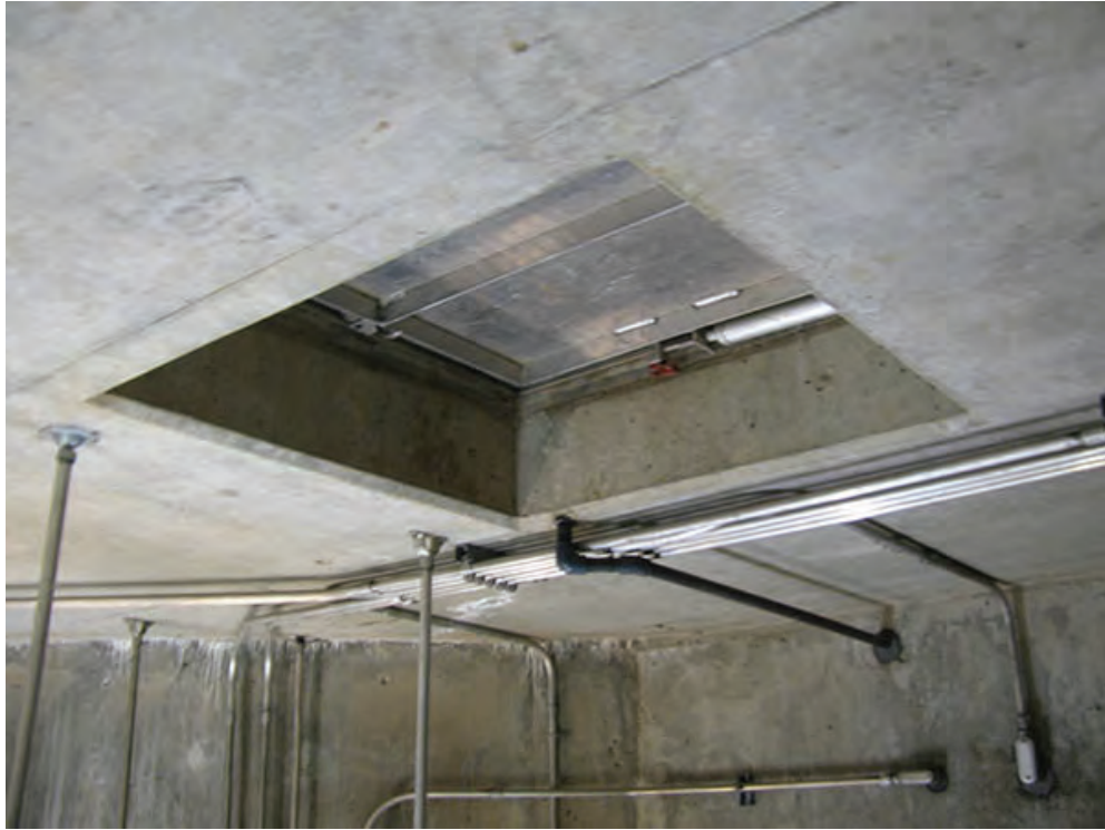
Photo 1 – LS1 – Access hatch at the Sludge Thickening PS as seen from the underside of the concrete deck
