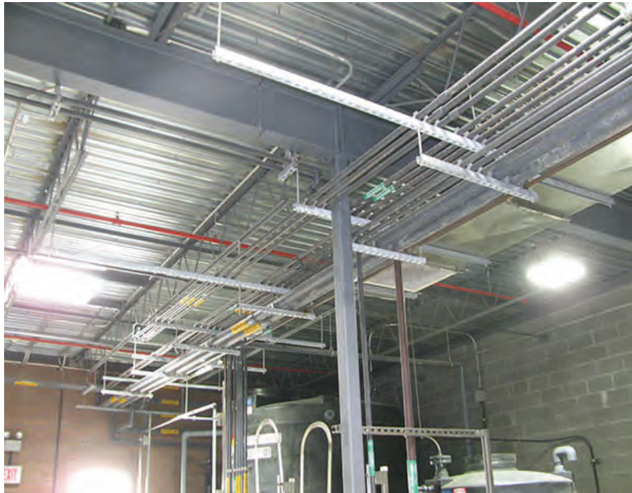
Photo 37 – S13 – The chemical piping at the Chemical Storage Room lacks transverse seismic bracing.
