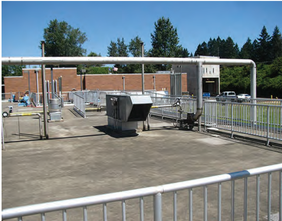
Photo 35 – S11 – The ozone destruct piping lacks seismic bracing at the top of the Ozonation Basin.
