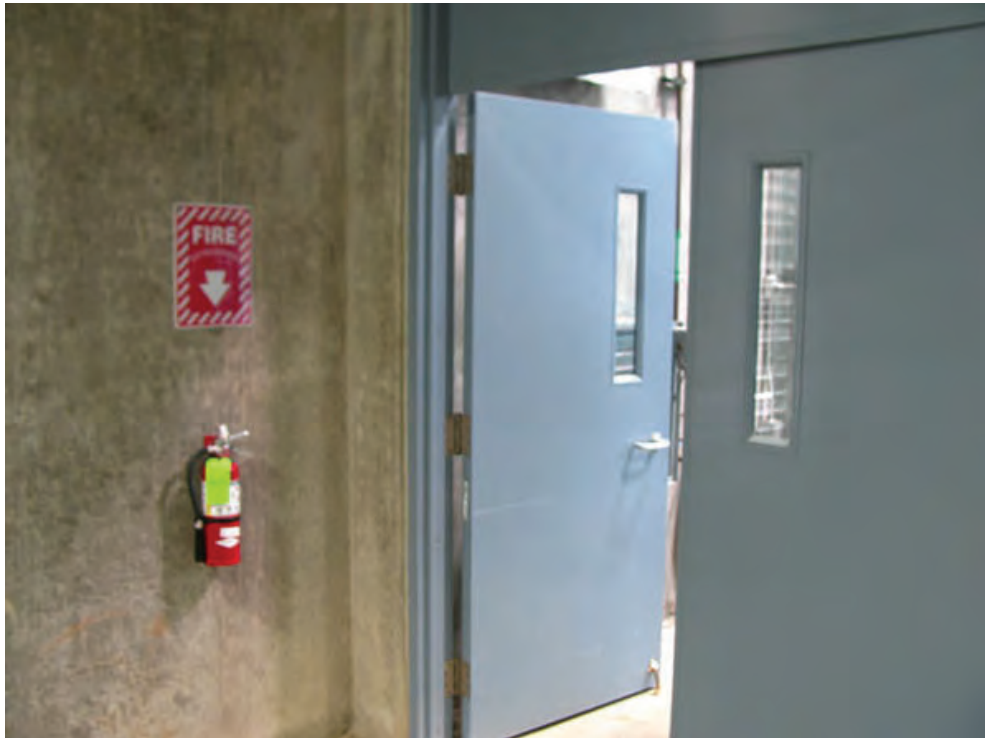
Photo 8 – LS4 – The Switchgear Room at the High Service Pump Station has electrical service rated at 1200 amps or higher requiring panic hardware on doors
