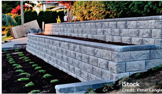
Tiered retaining wall with “horizontal offset” between lowest part and upper part(s) of wall
