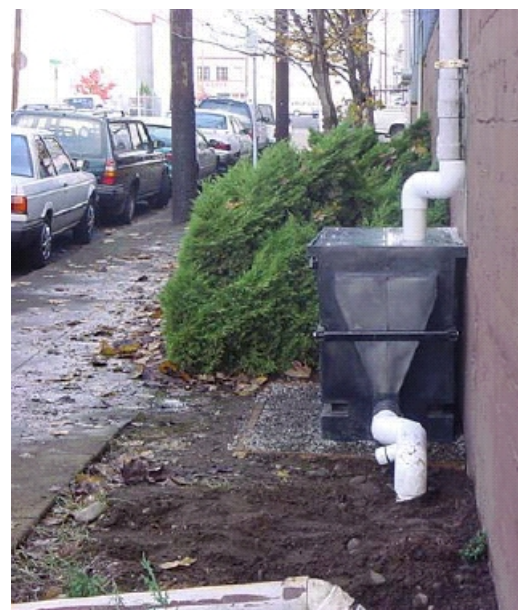
Roof Downspout type filter
