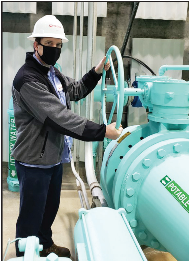
Veolia North America staff at Water Treatment Plant isolation valve.
