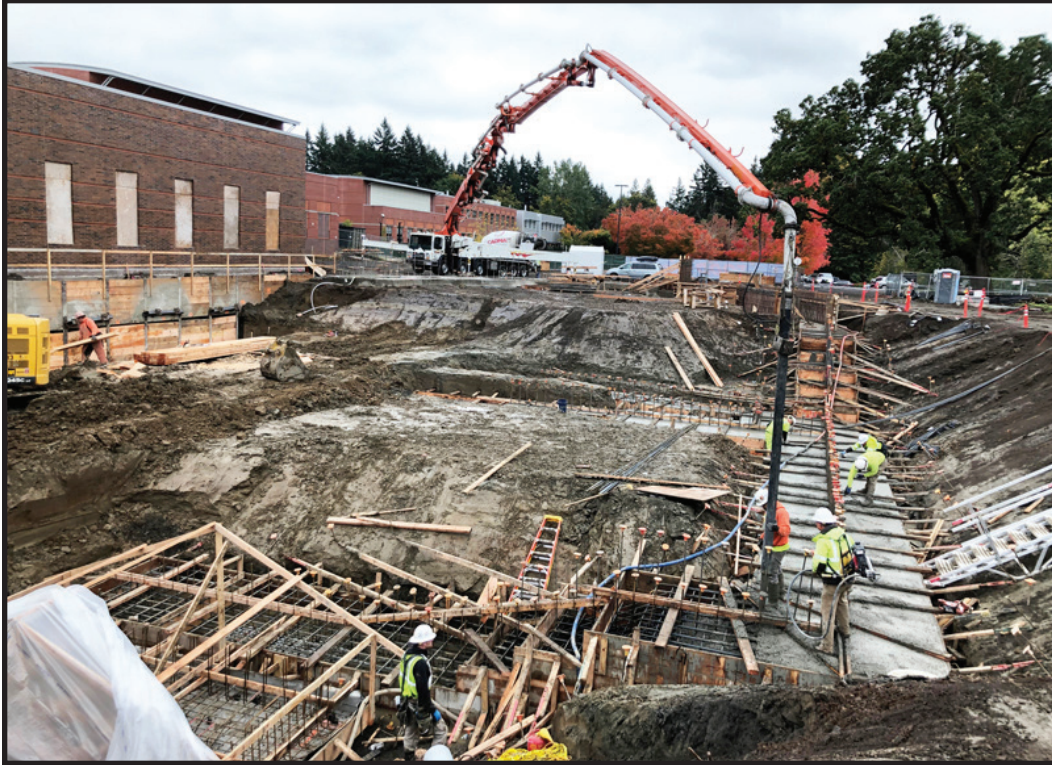
Pouring the footing for the Wilsonville High School Performing Arts Center expansion.
