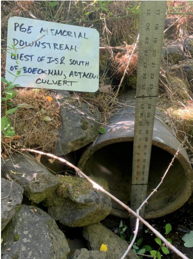
Photo 8: 14-inch cast iron pipe to well adjacent to culvert pictured in Photo 9. Located west of Interstate 5 and south of Boeckman Road.
