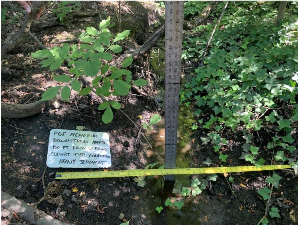
Photo 10.A: Facing NE downstream of unfound culvert in a wooded landscape. Typical conditions with heavy sediment and a water depth of 1.5-inches.
