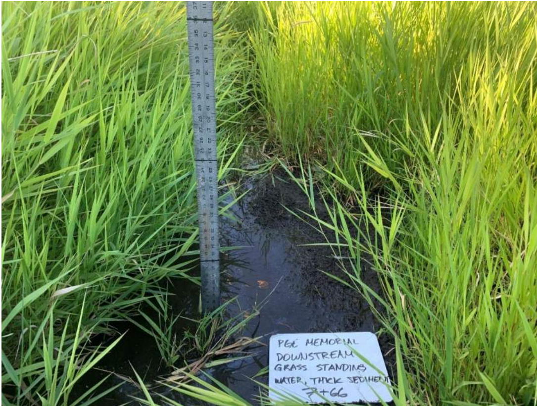
Photo 03: Downstream standing water depth of 4-inches with thick sediment and surrounding tall grass.
