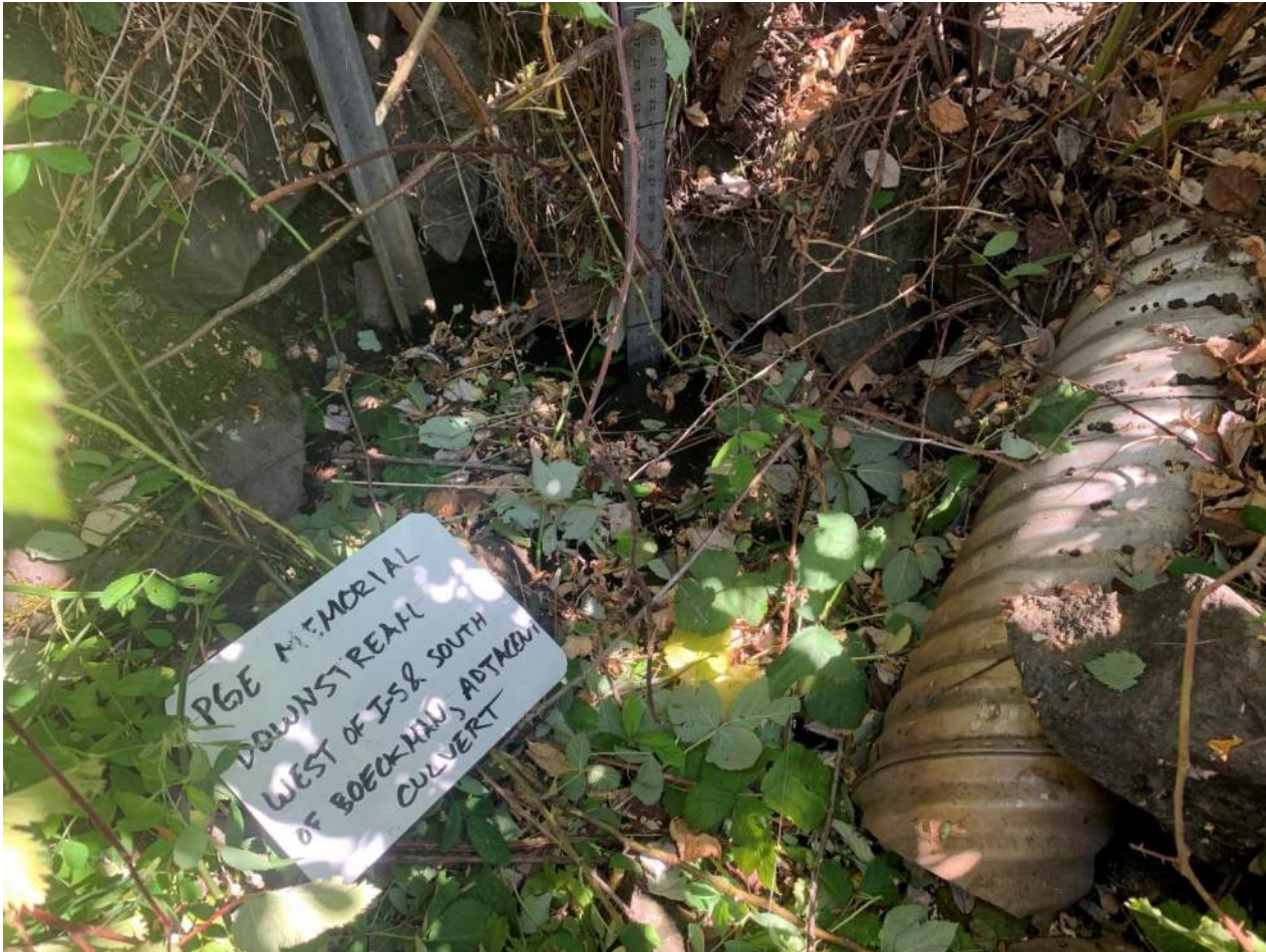
Photo 07: 18-inch Culvert partially crushed and with 10-inches of standing water. Located west of Interstate 5 and south of Boeckman Road
