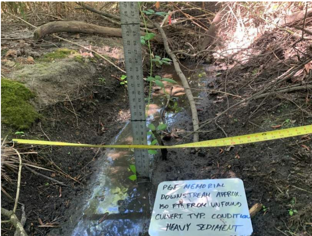
Photo 12.B: Facing SW downstream of unfound culvert in a wooded landscape. Typical conditions with heavy sediment and a water depth of 1-inch.
