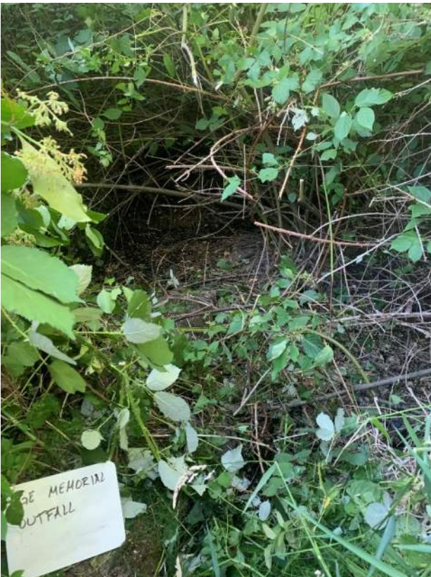
Photo 02: Culvert A 24-inch Not found. Heavily vegetated with tall grass, blackberry bushes, and other invasive species.
