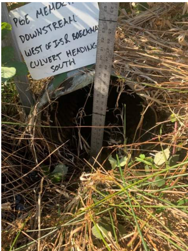
Photo 06: Heavily vegetated area surrounding 18-inch culvert heading south, located west of Interstate 5 and north of Boeckman Road.
