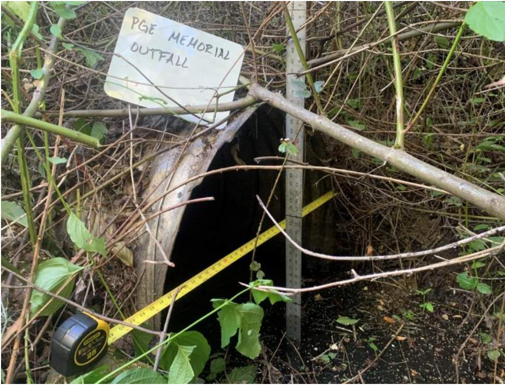
Photo 01: PGE Memorial 42-inch outfall with a 6.5-inch water depth.
