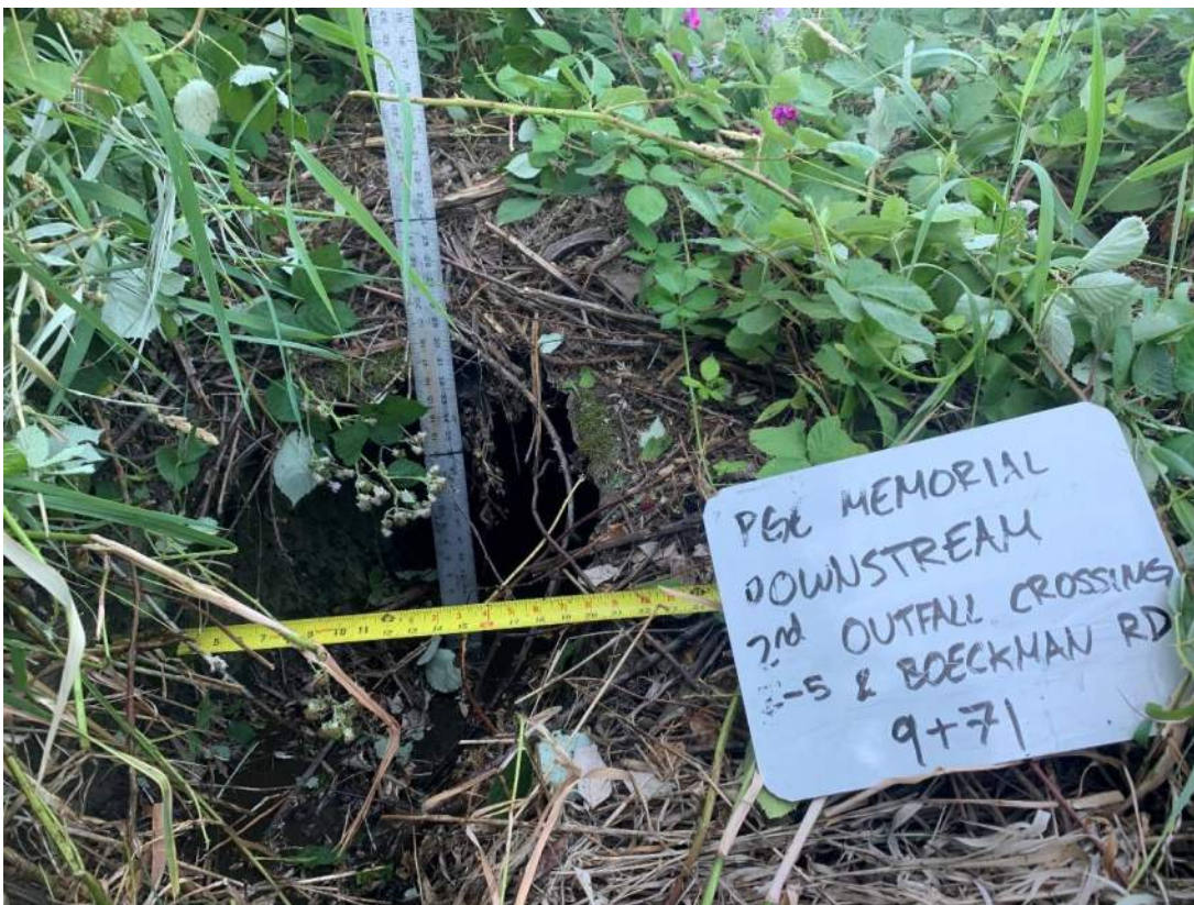
Photo 04: The heavily vegetated area surrounding 18-inch culvert B, located east of Interstate 5 and north of Boeckman Road.
