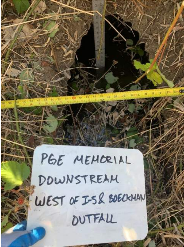
Photo 05: Overgrown invasive species surrounding 18-inch culvert B, located west of Interstate 5 and north of Boeckman Road.
