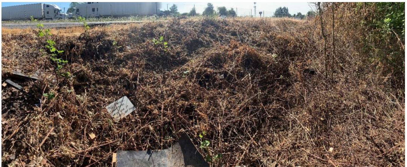
Photo 9: General location of unfound 24-inch A culvert. The area was surrounded by dry vegetation and other debris from the highway.
