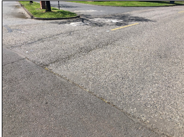
Photo 2: North Entrance Drive – Fatigue Cracking and Raveling. Note sealcoat on eastern section of roadway.
