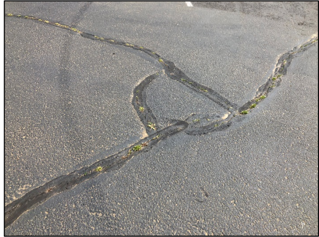
Photo 4: North Parking Bay – Crack Seal closeup
