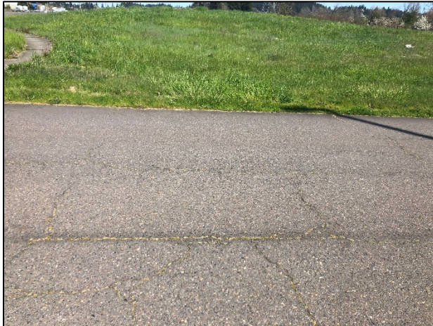
Photo 1: North Entrance Drive – Fatigue Cracking
