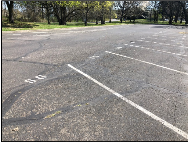
Photo 3: North Parking Bay –Random/ Transverse/ Longitudinal Cracking
