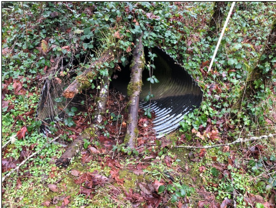
Emergency Overflow Culvert (42"x66" CMP - Corrugated Metal Pipe) Located on Upper Bench
