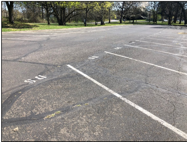
Photo 3: North Parking Bay –Random/ Transverse/ Longitudinal Cracking
