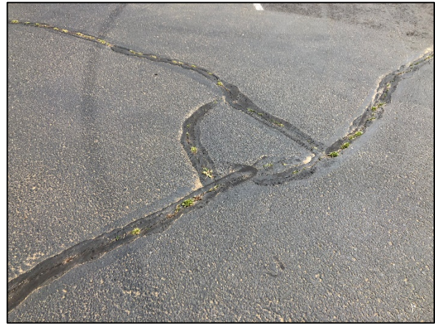
Photo 4: North Parking Bay – Crack Seal closeup
