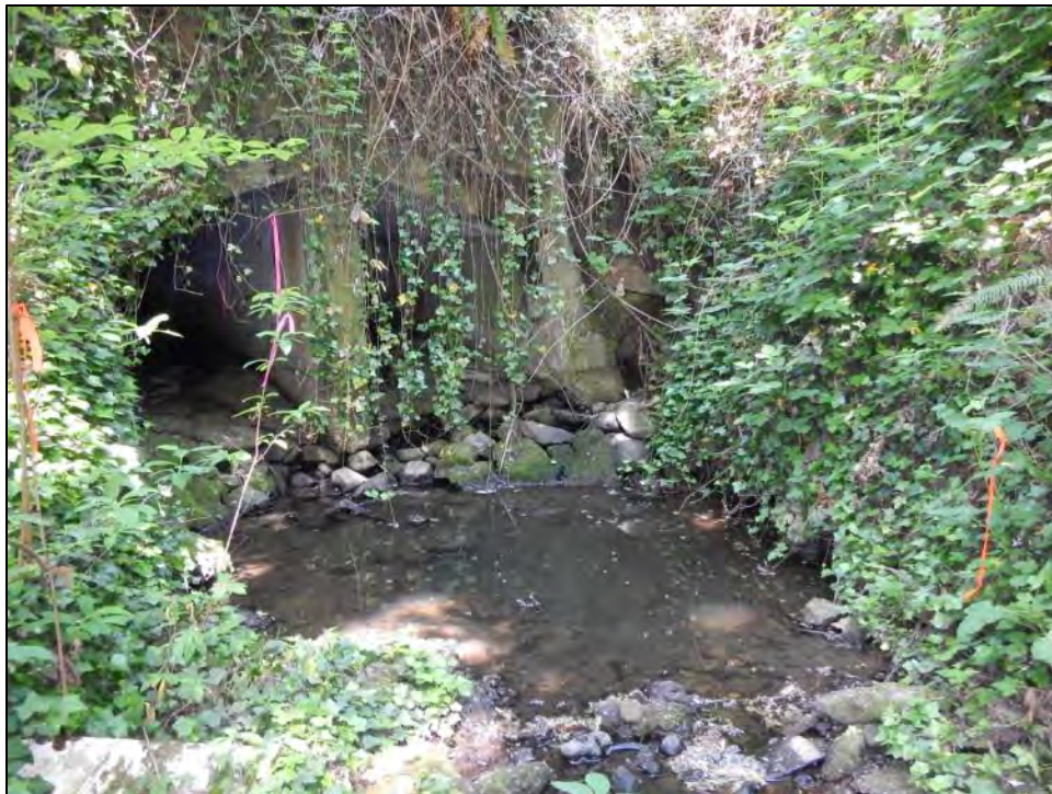
Photo 3: Looking northwest at box culvert where Arrowhead Creek enters the west end of study area (May 8, 2015). OHWM lies at the base of the shrubs marked with the orange flags.
