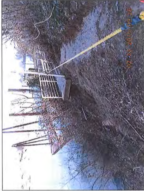
Photo 5. Existing path were landslide occurred, blocking access to existing gangway and landing platform. View northeast. Photo: Pioneer Group, February 22, 2015.
