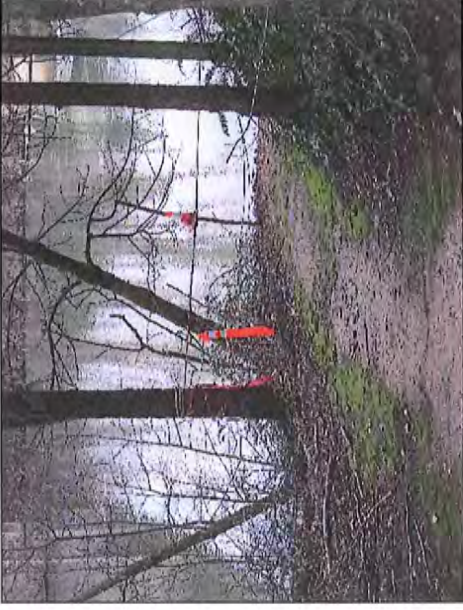
Photo 3. Existing pathway in ODOT ROW to be restored. Landslide occurred just beyond the orange cone. View north. Photo: Pioneer Group, February 22, 2015.
