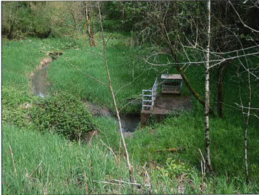
Photo W. View south of Boeckman Creek and concrete drain structure. Photo date April 18, 2017.
