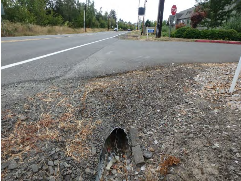
Figure 11. Pipe under church driveway is 10 inch corrugated metal at upstream end and 8 inch plastic at downstream end (Node 27).
