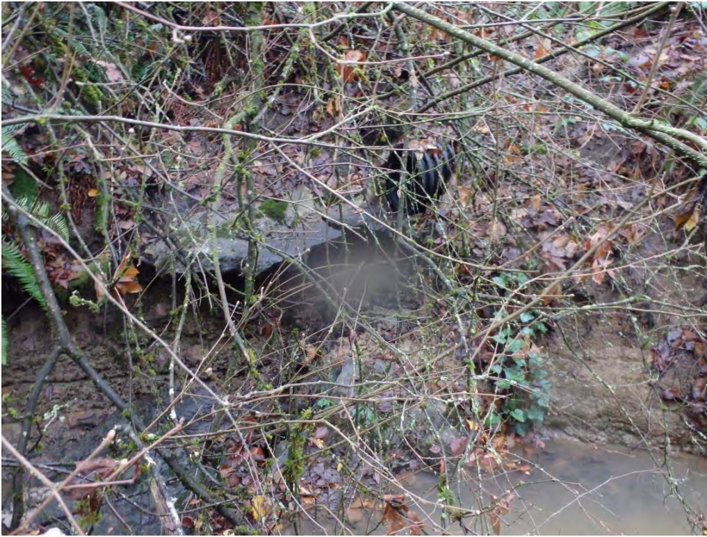
Photo 16 Perched Culvert on Right Bank
