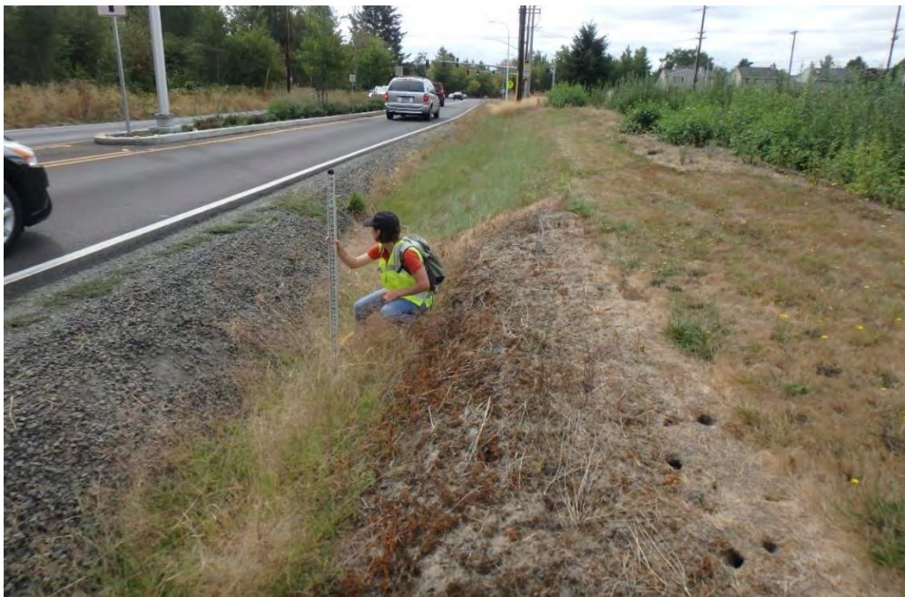
Figure 12. West ditch left bank 2.5 ft high and right bank grassed 3 ft high with transition from 1:1 side slope to 2:1 side slope (Node 31).
