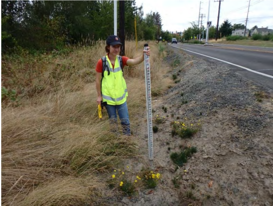
Figure 5. East ditch with sloughing from right bank 2.5 ft height and bottom 2.75 ft width. (node 7)
