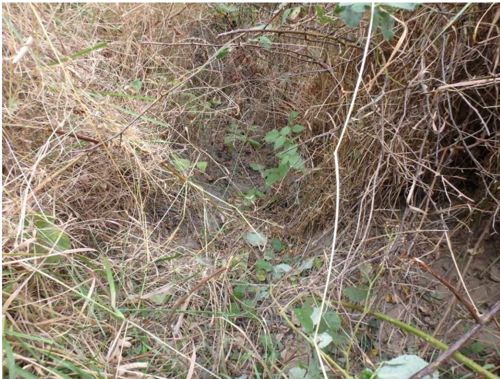
Figure 2. East ditch at outlet of 15" culvert (node 3). Gravelly bottom and heavily vegetated 2:1 side slopes. Roadside right bank 3ft height and left bank 2.5ft height.
