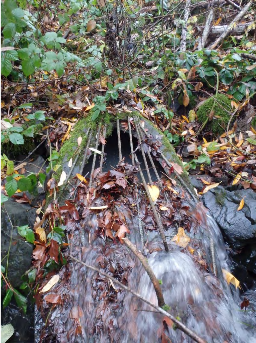
Photo 9 24-inch Outfall from energy dissipation Concrete Box at outfall from 36-inch Pipe
