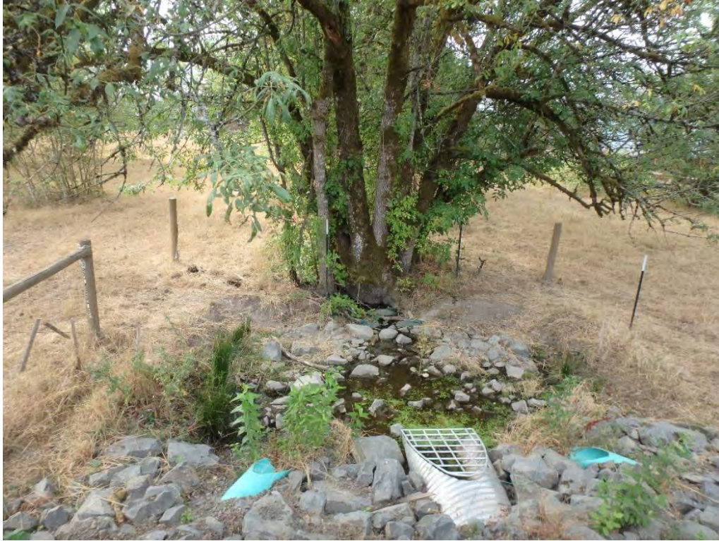
Figure 15. Outlet of 24" Culvert south of SW Advance Rd (Node 14)
