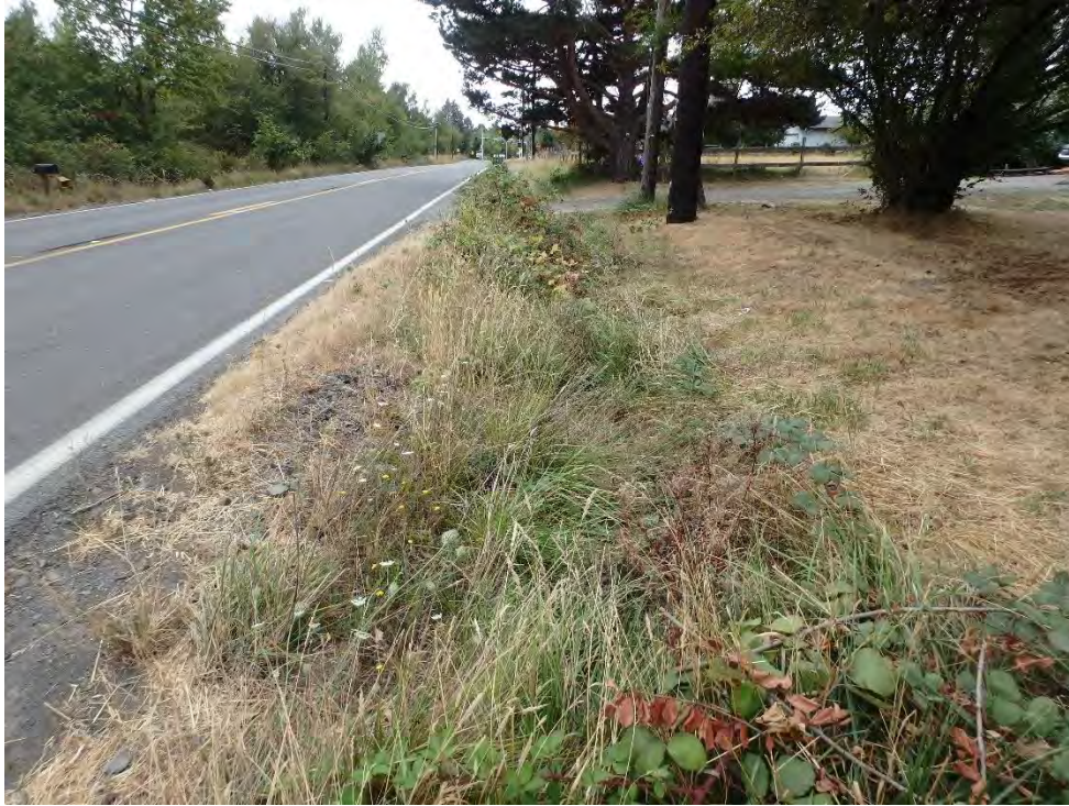
Figure 9. West ditch downstream of 15 inch cross culvert, 2 ft depth, 1.5 ft bottom width and densely vegetated 2:1 side slopes, crosses 4 driveways in 12 inch culverts (Node 21).
