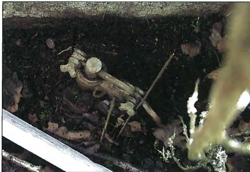
Figure 16. Valve at the base of the trough.
