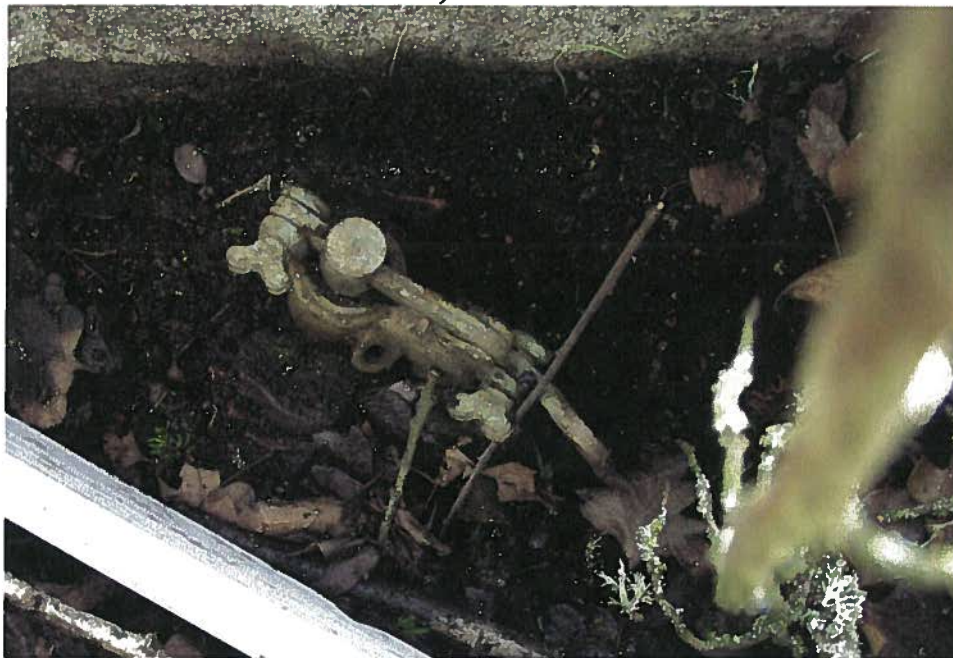
Valve at the base of the trough.
