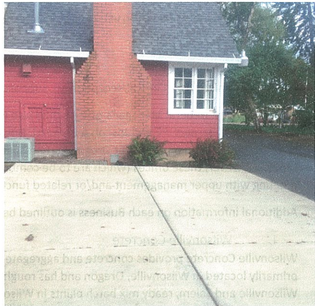
Figure 10. Concrete Parking pad for ADA Space
