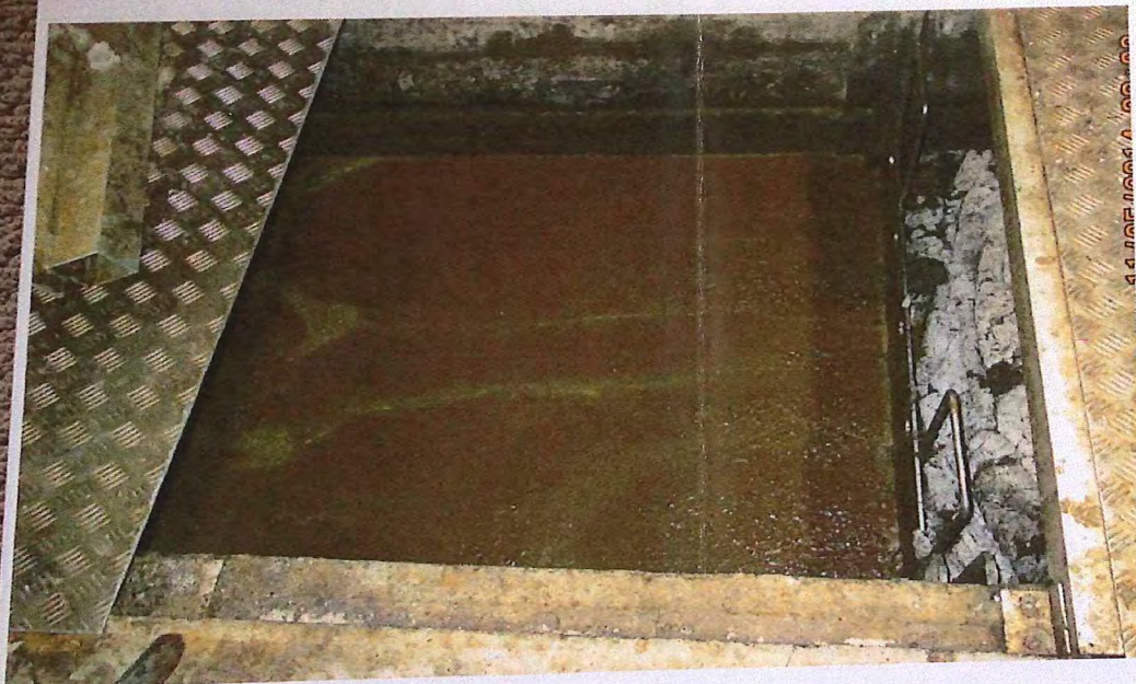
De-packaged organics prepared for pumping into Anaerobic Digester
