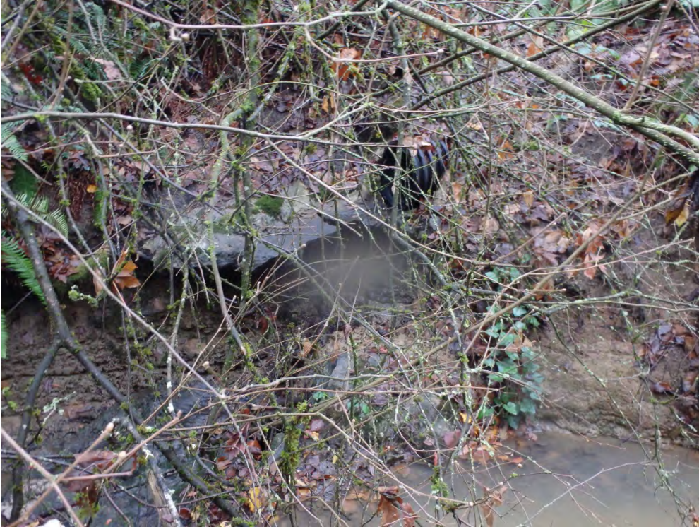
Photo 16 Perched Culvert on Right Bank
