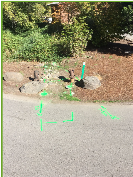
Showing the layout of the pipes
