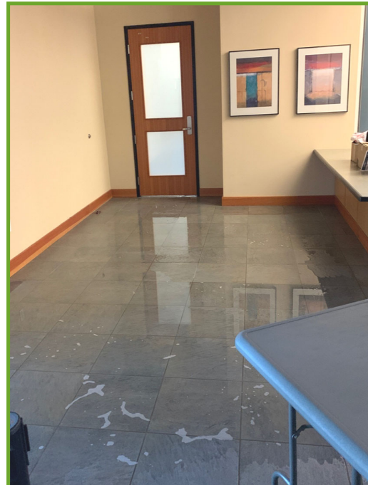
Massive puddle at the front desk
