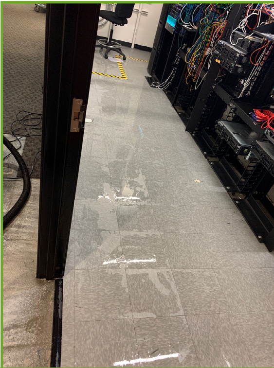
Computer server room— safe but just barely
