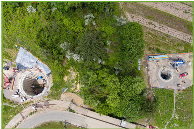
Launch shaft on the left and receiving shaft on the right for the trenchless crossing of Arrowhead Creek
