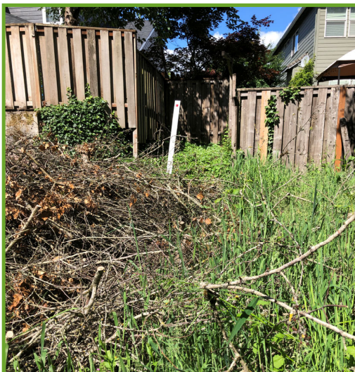
Outfall obscured by tree debris
