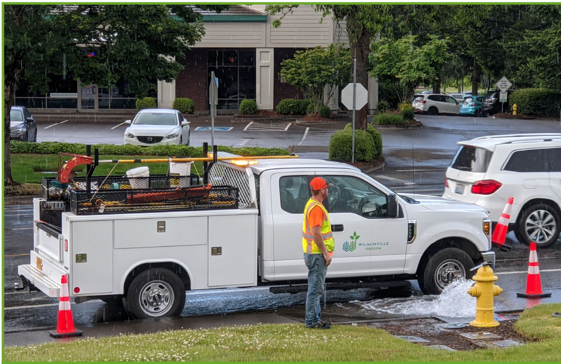
Hydrant flushing outside Public Works
