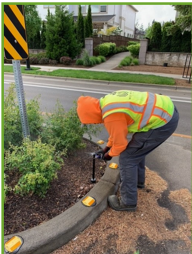
Sprinkler head adjustment
