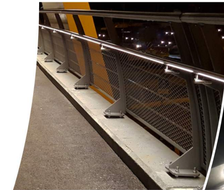
Continuous Handrail Lighting
