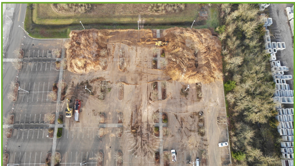
After —Chips remaining at the debris site looking to the west
