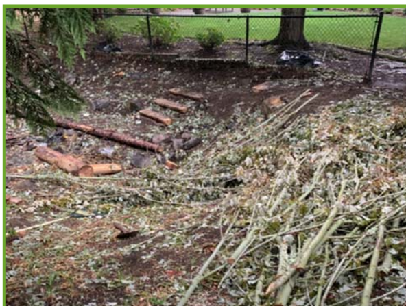
Debris in detention pond
