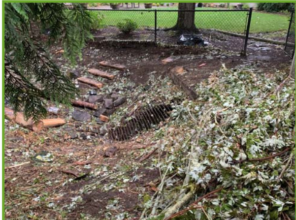
There's a grate under there!
