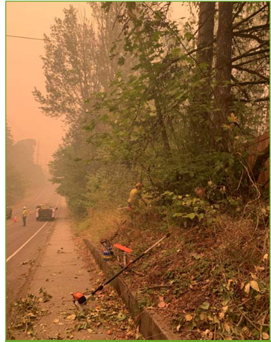
Clearing potential hazards
