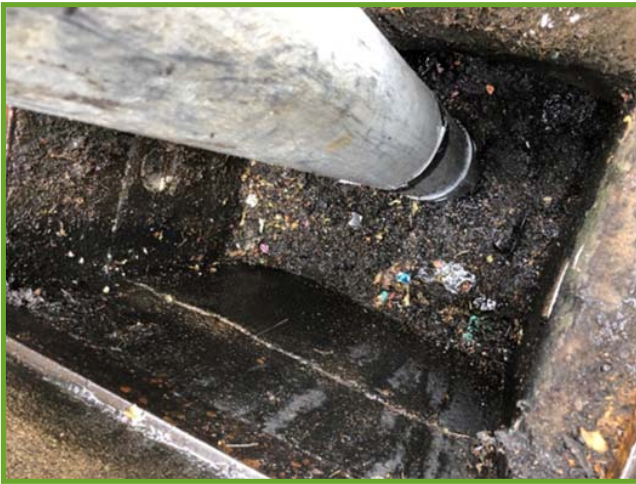
Before—no pipe in sight
