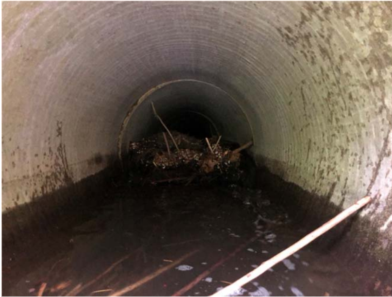
Beaver's dam inside a stormwater pipe
