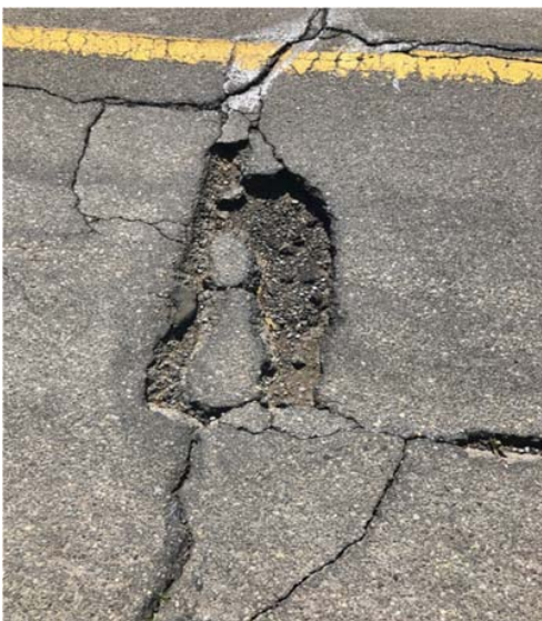
Pothole before being fixed
