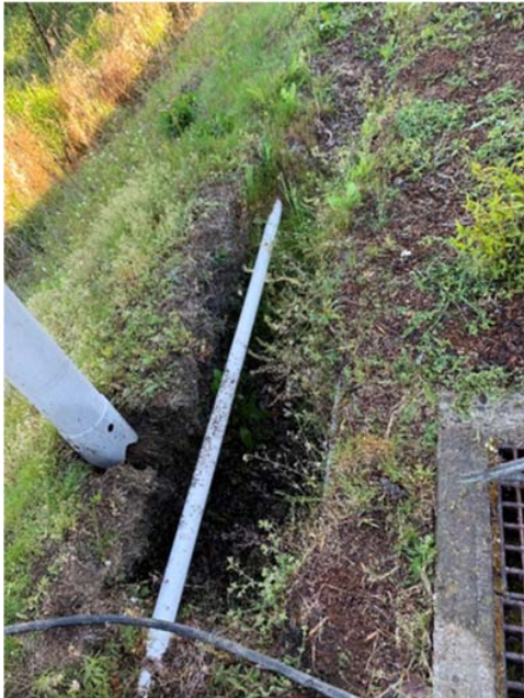
Sink hole along Boeckman Road
