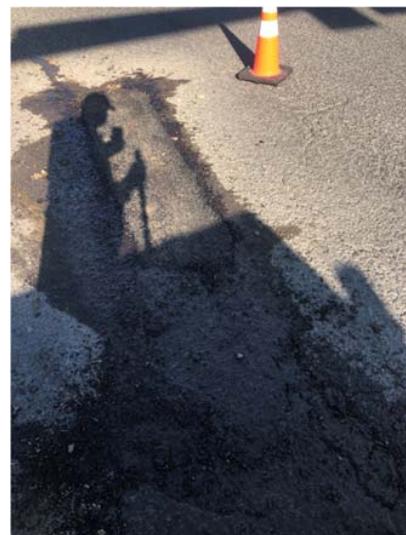
Pothole after repair
