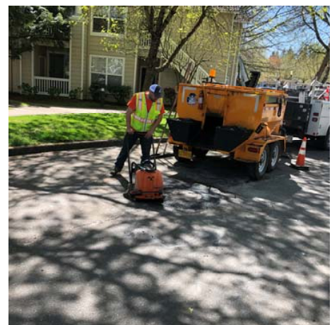
Asphalt patch around casing ring
