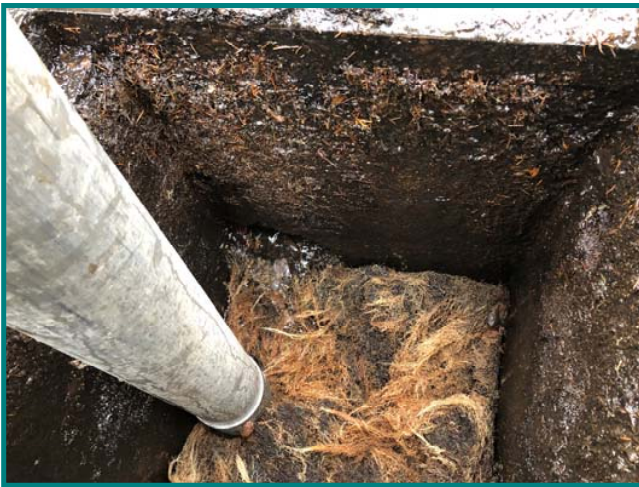
Stormwater Maintenance Specialists Jay Herber and Randy Burnham clear a root engulfed catch basin with the vector
