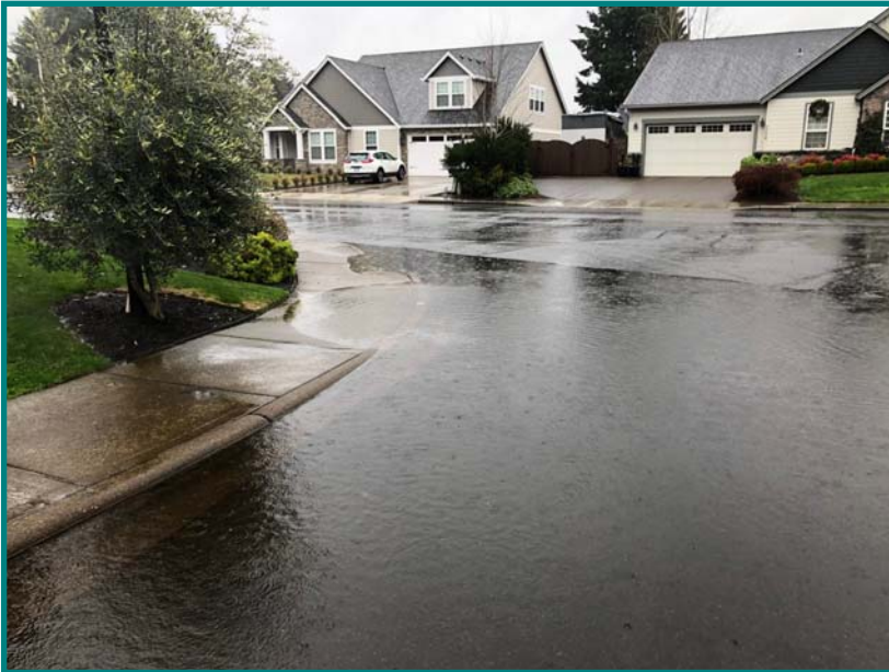
Known problem with localized road flooding due to leaves accumulating over the stormwater grate
