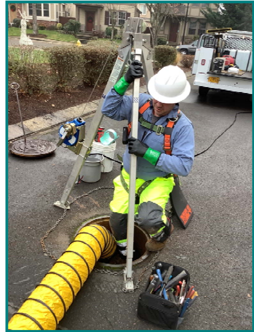
Kyle Bean—Entering Manhole (Confined Space)
