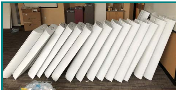
Old lighting fixtures
