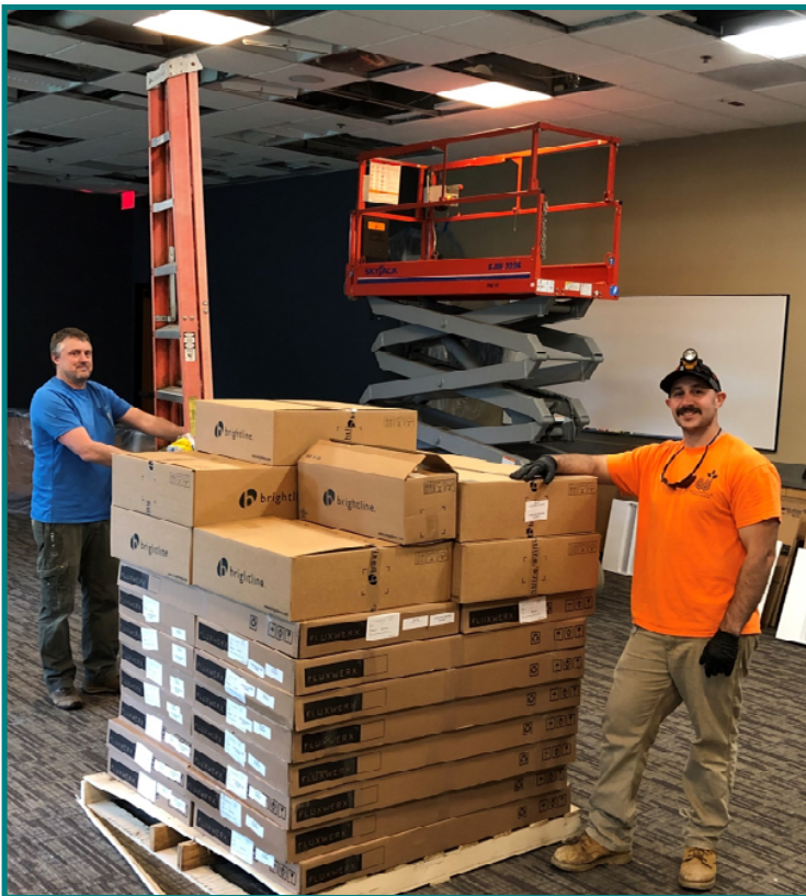
Chris, ECO Electric and Javid, Facilities
