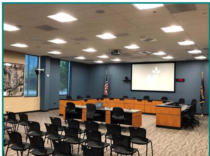
After (LED lights) - Council Chambers
