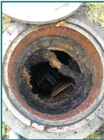
Left: Root intrusion in an old manhole.
