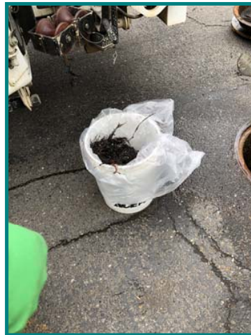
Left: Roots removed from sewer manhole.
