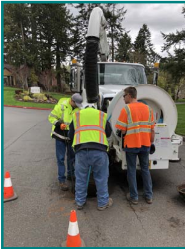
Left: Acting Water Tech Sam Kinnaman receives cross training from Sewer crew members Paul Havens and Paul Walker on how to jet sewer lines.
