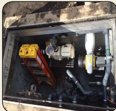
Upgraded Sofia Park pond electrical components to improve efficiency of operations
