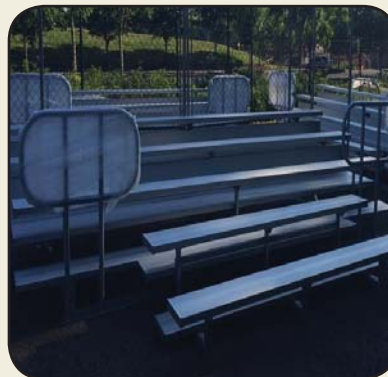
Received delivery and began construction of five ADA compliant bleachers for Memorial Park
