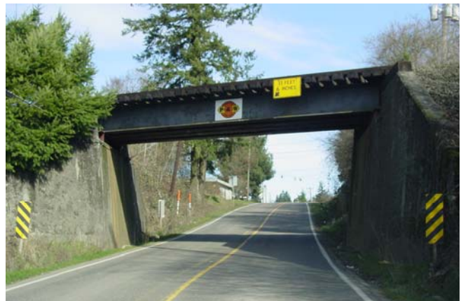
The railroad bridge over Grahams Ferry Road has limited horizontal and vertical clearance. This creates a safety hazard, particularly for bicyclists, pedestrians, and freight traffic.
