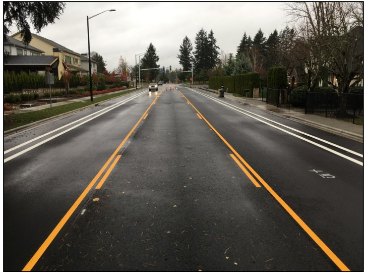
Tooze Road, looking west to new traffic signal at Grahams Ferry Road.
