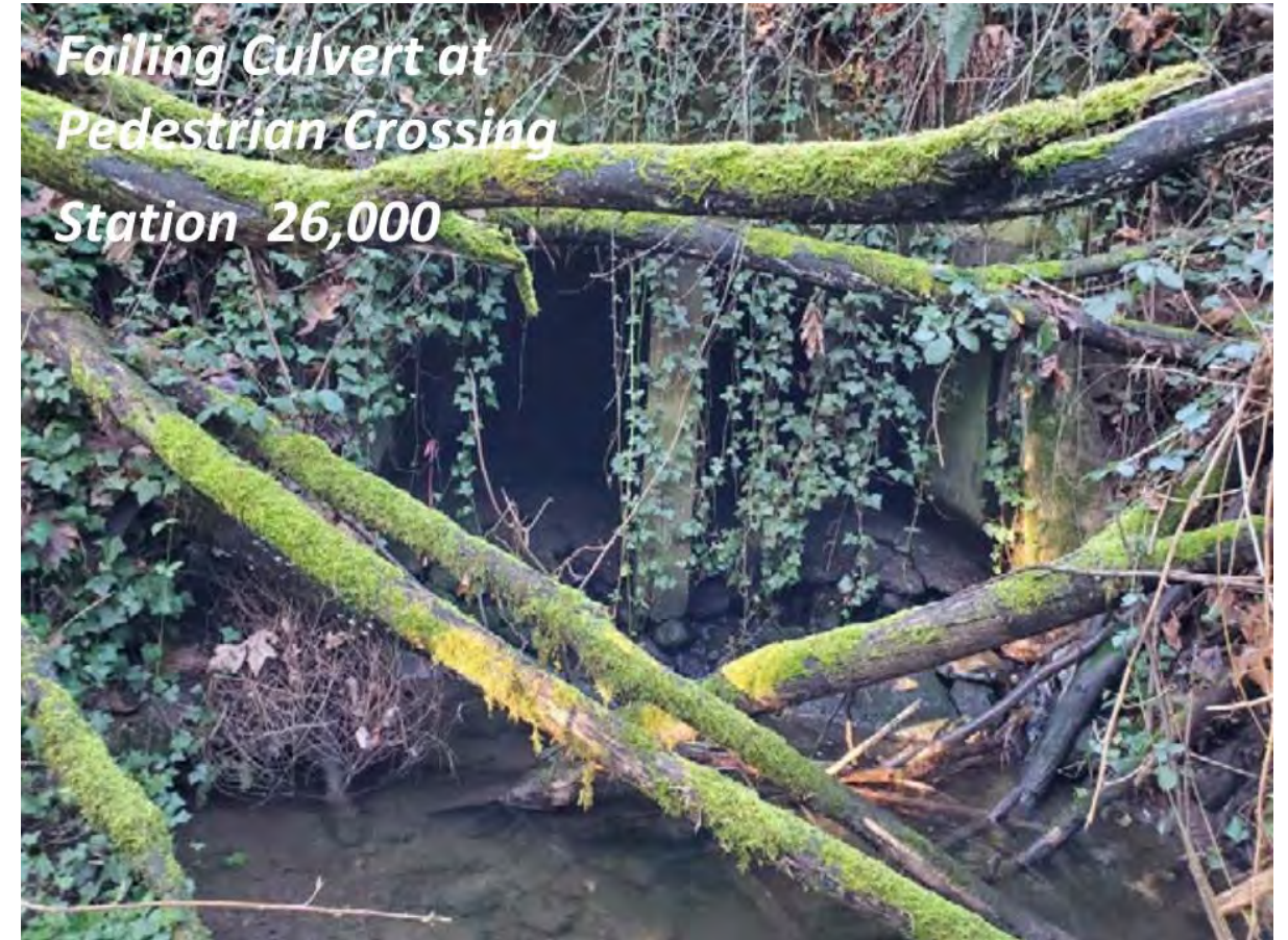
Falling twin 5 ft x 5 ft culverts under pedestrian crossing looking upstream (Source: Geomorphic Stream Assessment, Waterways Consulting, May 2022)
