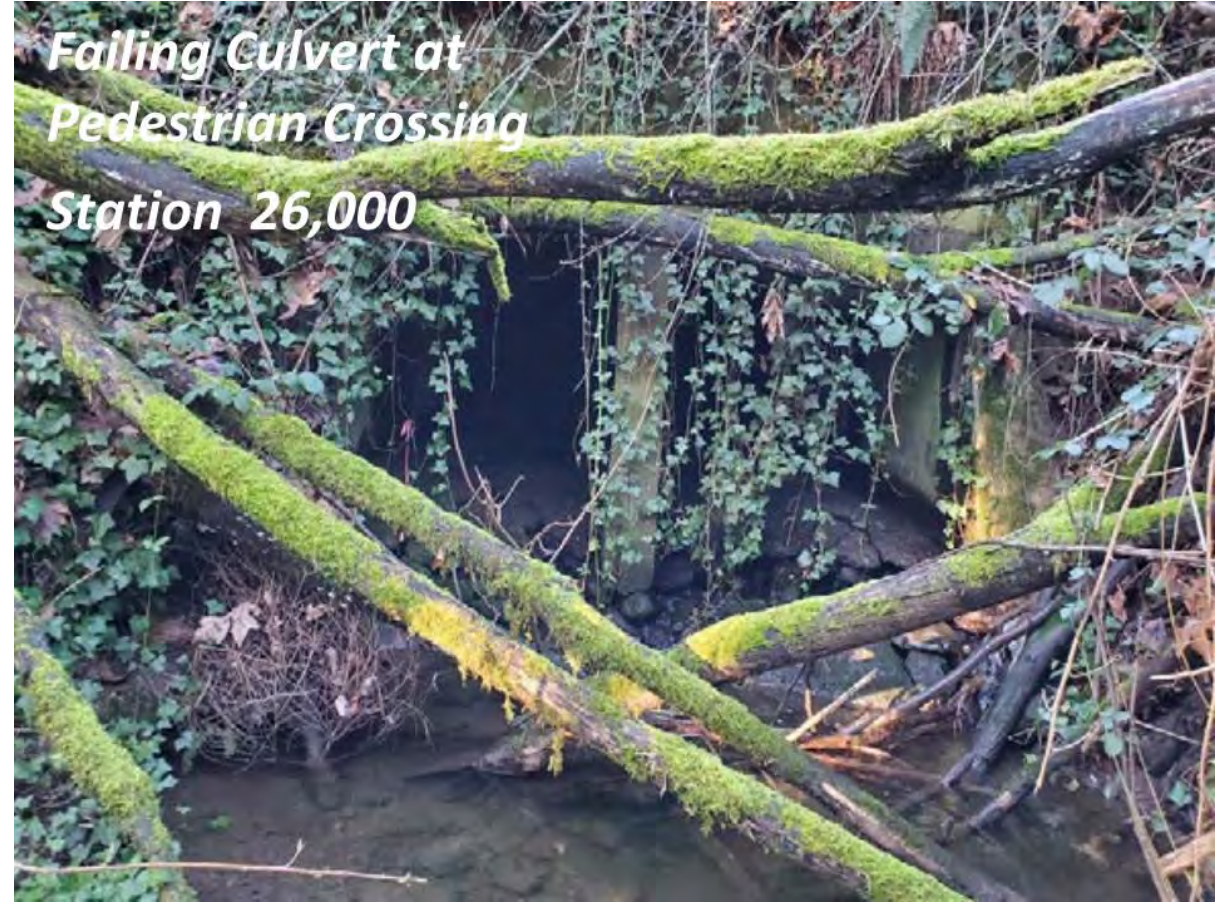
Falling twin 5 ft x 5 ft culverts under pedestrian crossing looking upstream (Source: Geomorphic Stream Assessment, Waterways Consulting, May 2022)
