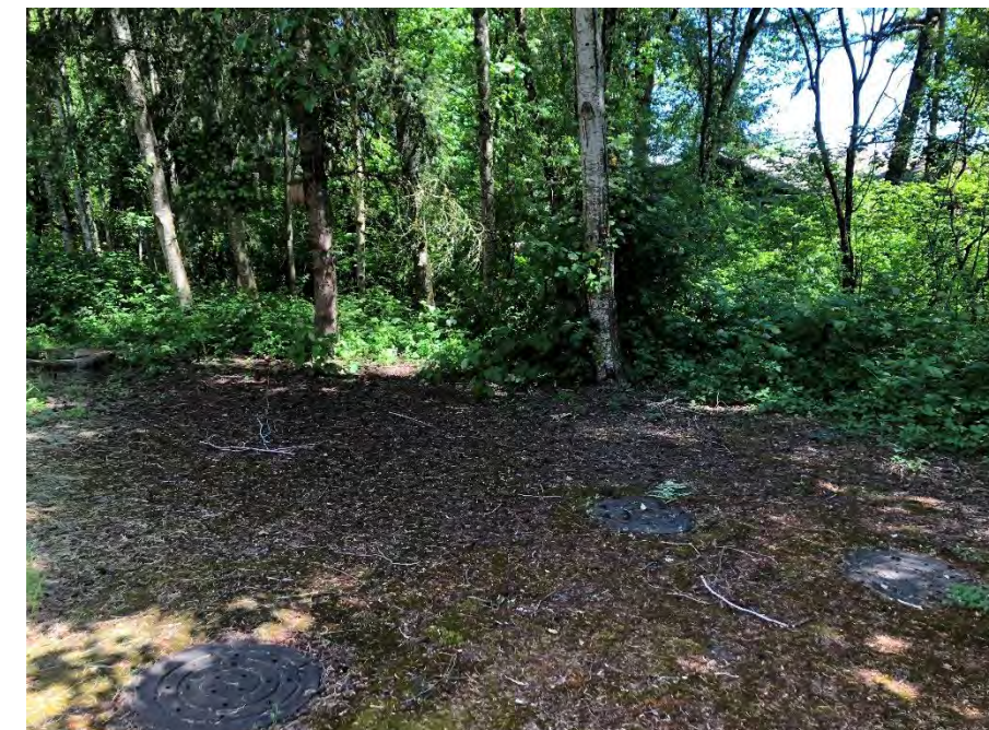
Upstream detention pipes location (May 2023)
