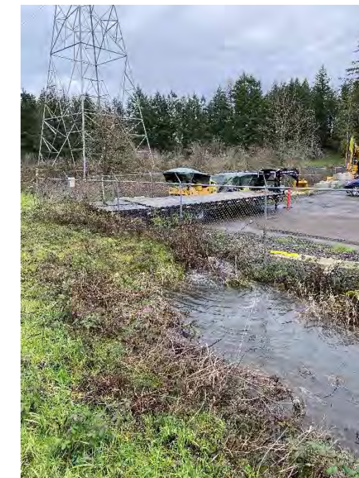
Conveyance channel and impoundment south of Day Road after storm (Jan 2022)
