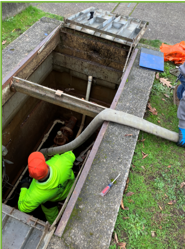
Accessing a commercial meter
