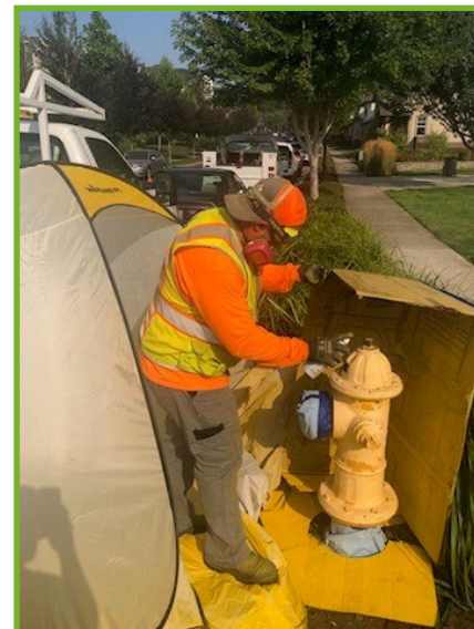
Spraying the hydrant
