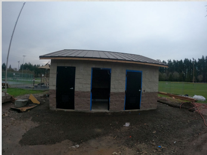
Restroom Awaiting A Sidewalk
