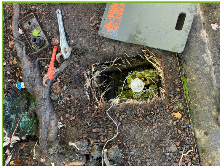
Roots growing around the meter box
