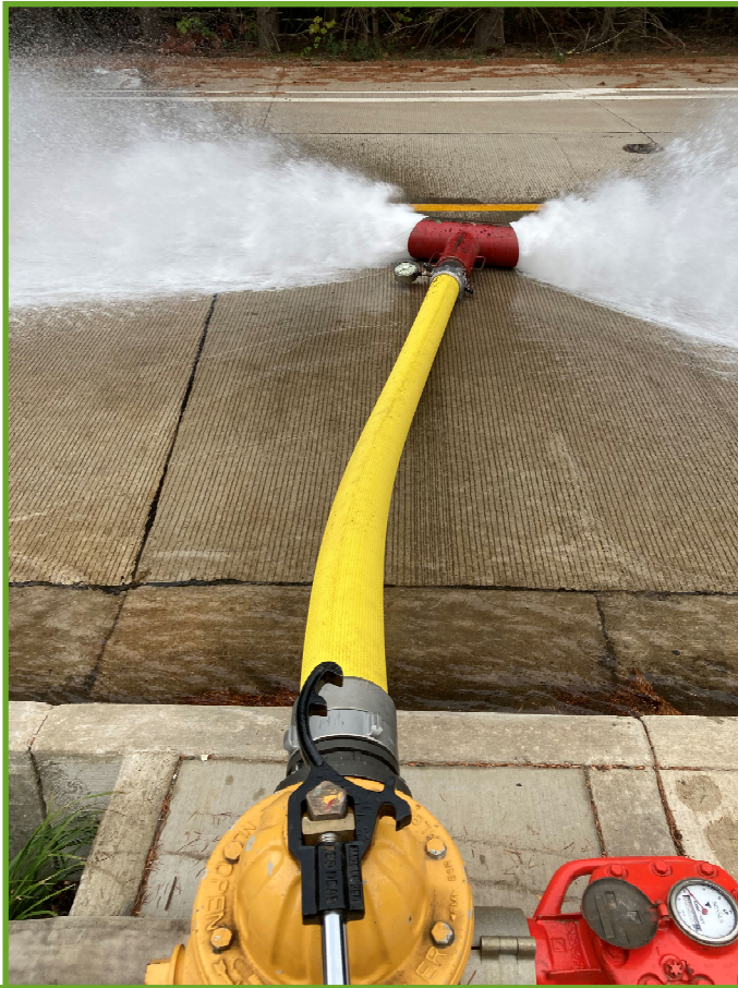
Hydrant open during testing
