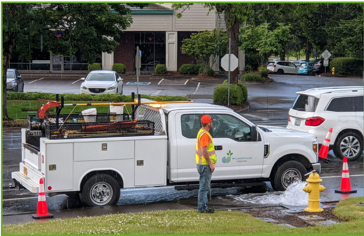
Hydrant flushing outside Public Works
