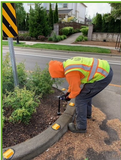
Sprinkler head adjustment
