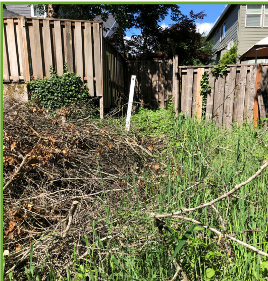
Outfall obscured by tree debris
