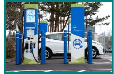
Example of a Charging Station
