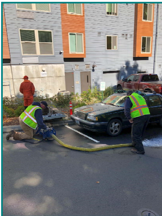
Steve Gering and Jerry Anderson, Water Technicians flowing water through a meter for testing.
