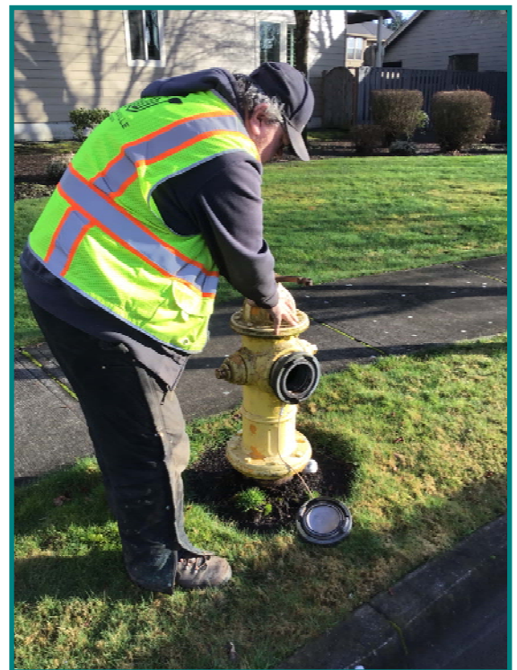
Water Distribution Technician Jerry Anderson performing a Hydrant Inspection
