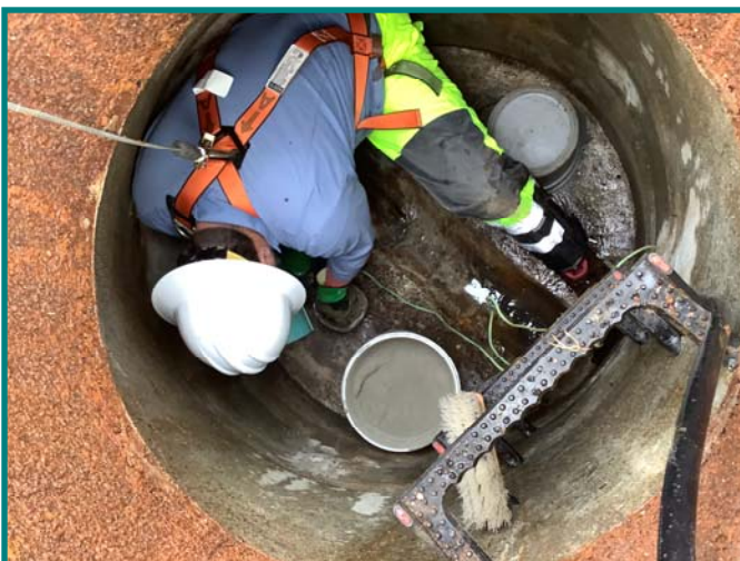
Kyle Bean — Inside the Manhole
