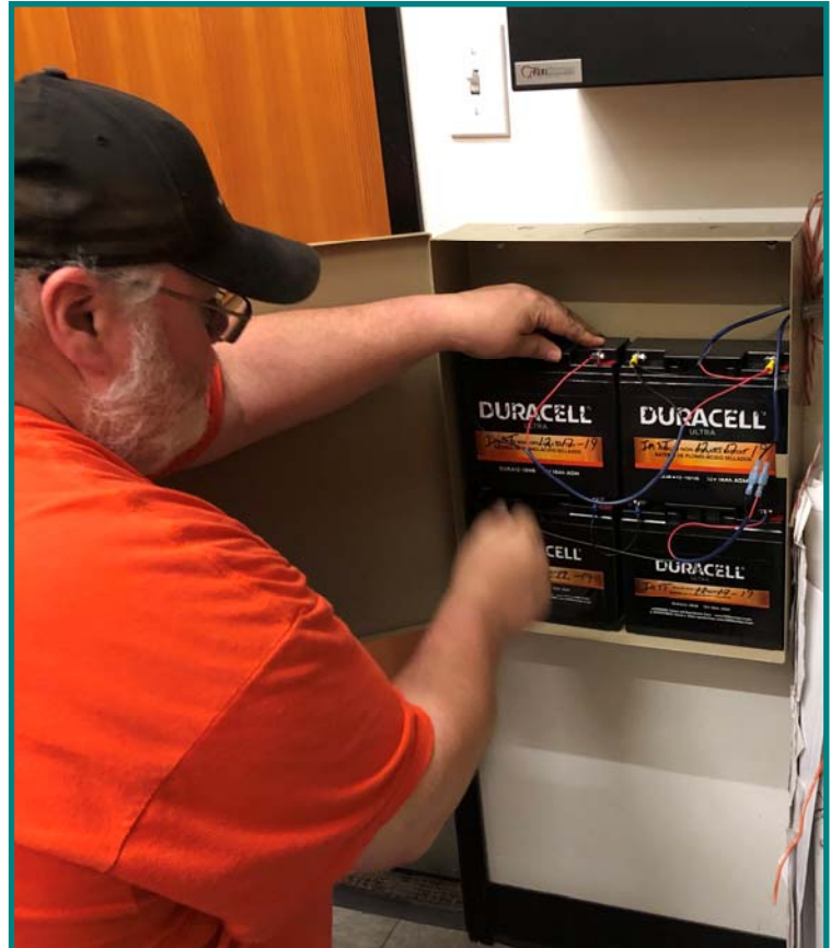
Robert Todd Checking Batteries
