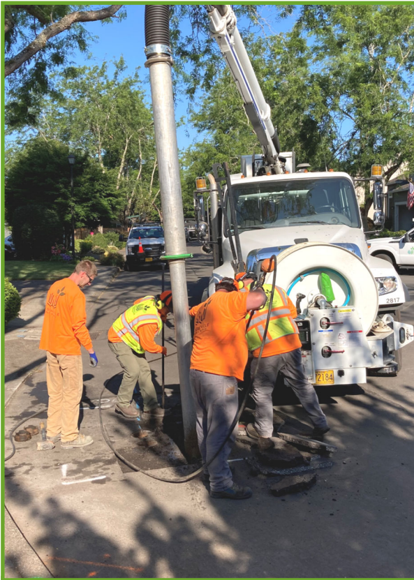
Accessing the blow off valve
