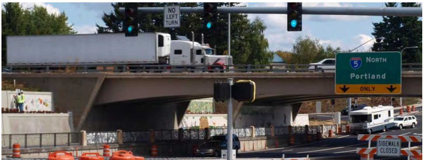
Student-produced artistic tiles being installed at the I-5/Wilsonville Road interchange underpass area, August 2012.
